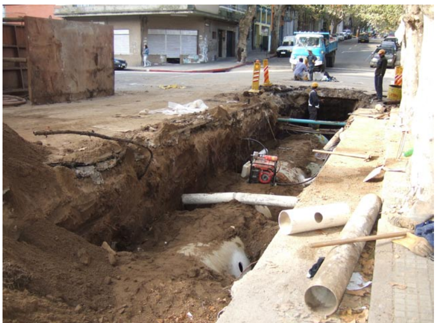
Fig. 20.22 The sub-surface of any street can be a complicated environment, creating uncertainty in full construction costs. Photo by Lloyd Wright
