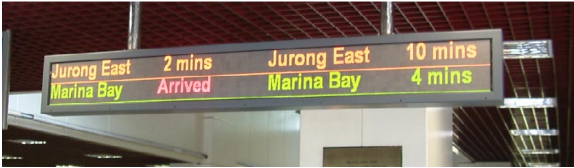
Fig. 12.73 In Singapore, customers can view arrival times prior to entering the platform area. Photo by Lloyd Wright
