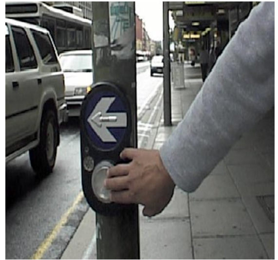
Fig. 13.85 A vibro-tactile pushbutton for requesting a crossing phase.
