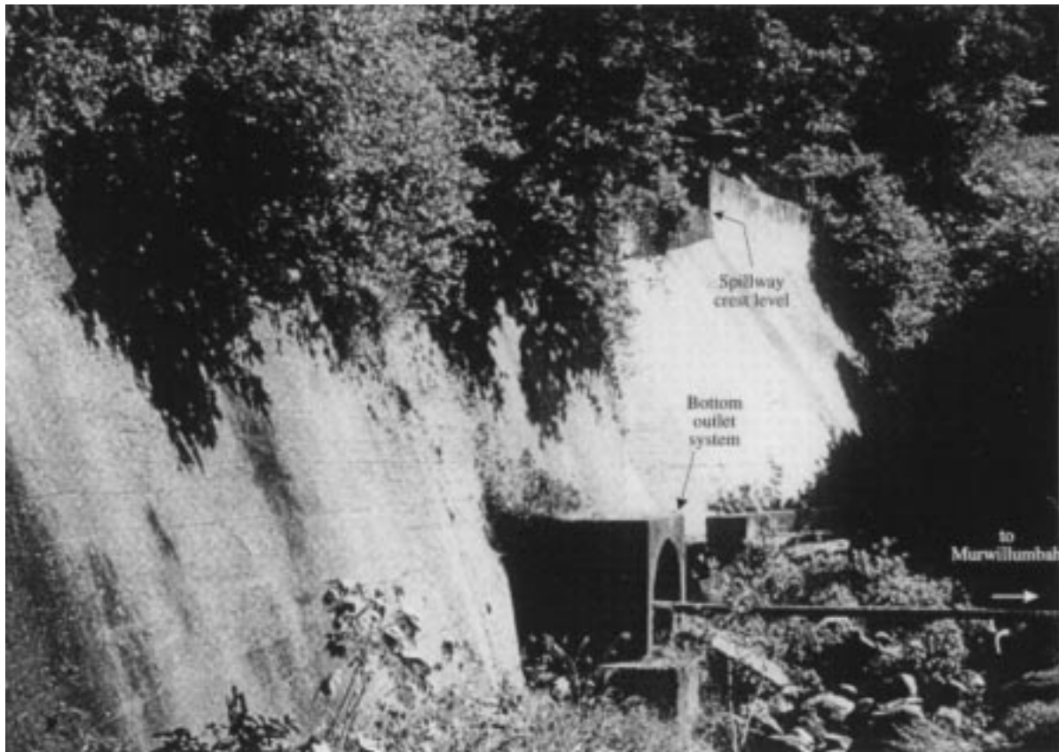
Fig. 5. Photograph of the Korrumbyn Creek Dam wall and the surrounding tropical rain forest. Photograph taken on 25 April 1997 (by H. Chanson).
