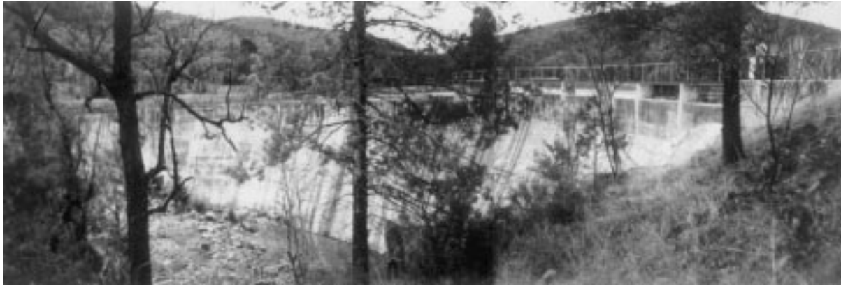
Fig. 6. Photograph of the Quipolly Dam, from the right bank. Photograph taken on 13 June 1997 (by H. Chanson).
