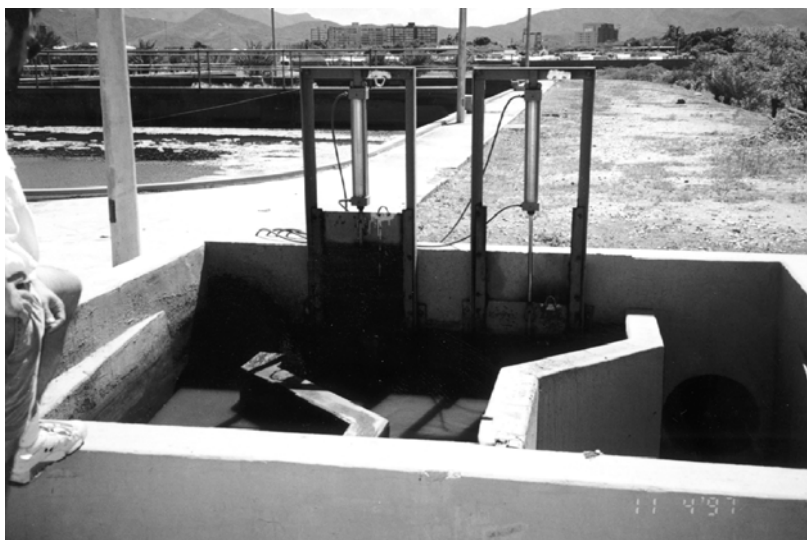
Simple pneumatically operated gates cyclically feed different zones of the MSBR at the Juangriego treatment plant.
