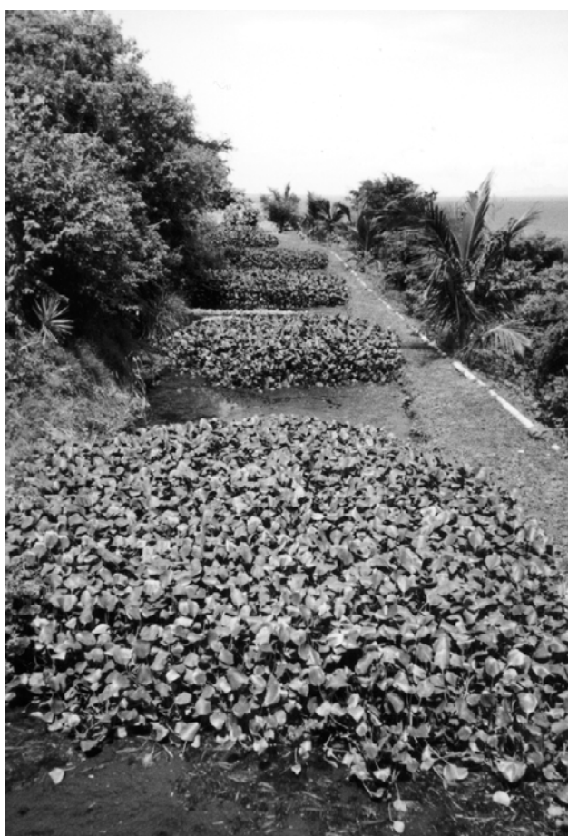
Constructed wetlands in a package treatment plant serving a hotel in St. Lucia.
