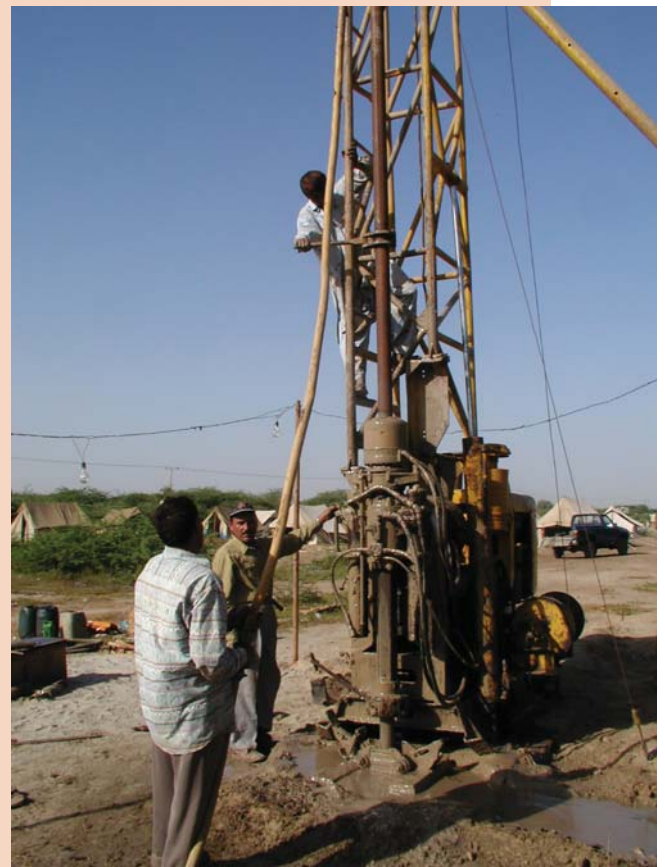
Drilling rig operated by the Geological Survey of Pakistan drills the flood plain of the Indus at Thatta, close to the modern river mouth.
