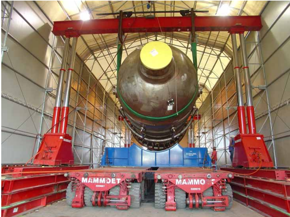
FIG. 25. Typical SG preparation facilities.
