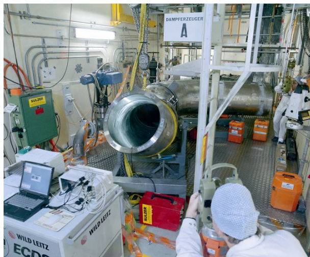
FIG. 41. New RCL pipe spool, welding already completed on-site, during 3-D topometry inspection ready for transportation to its welding position.
