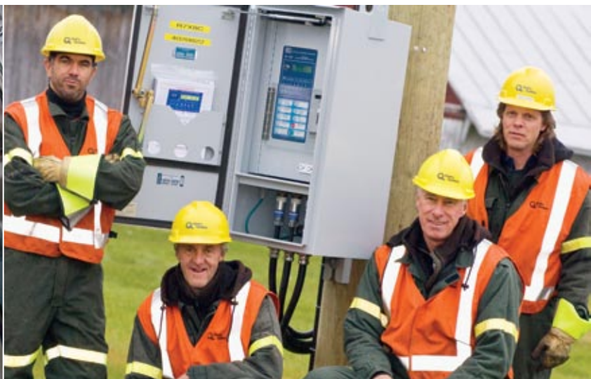
Line workers François Pelletier (left) and Jean Turcotte (right), and line crew chiefs Jean Ouimet and Denis Morin (centre left and centre right), pose in front of a control panel they installed as part of the distribution system automation program.
