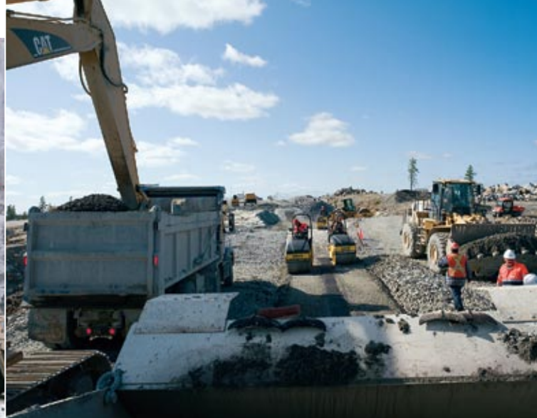
Construction of Nemiscau-1 dam. In a North American first, the dam was made watertight with an asphalt concrete core.
