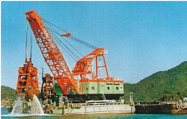
Fig. 5. The dredge that has to operate alongside the ship traffic in the Bosphorus.
