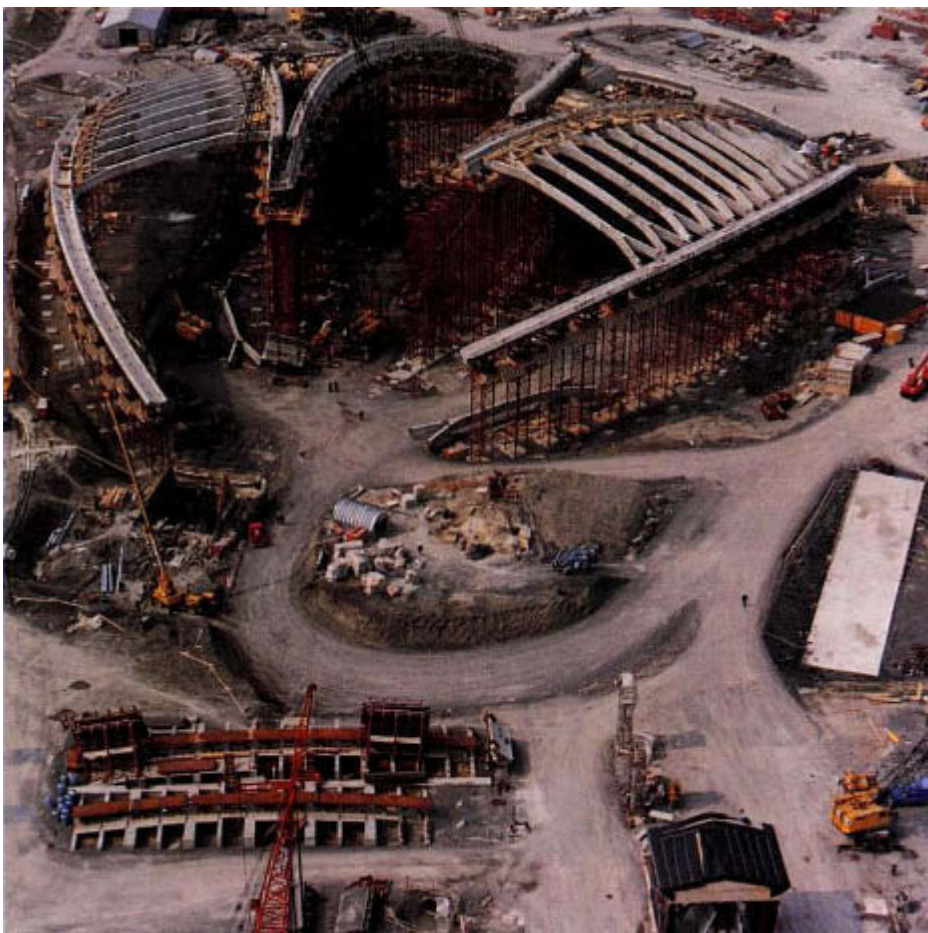
The Olympic Velodrome in June, 1974. Approximately 60 percent of the prefabricated voussoirs are in place on the scaffolding.
