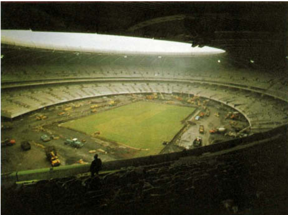
In April, 1976, work starts on laying turf inside the Olympic Stadium while preparations are made to remove the heavy equipment.
