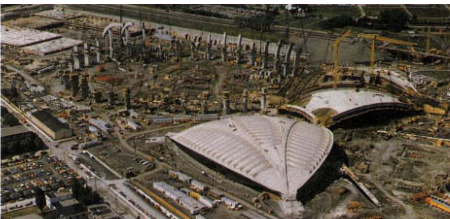
Work progress at the Olympic Park. From top to bottom: October 4, 1974; March 14, 1975; July 22, 1975.
