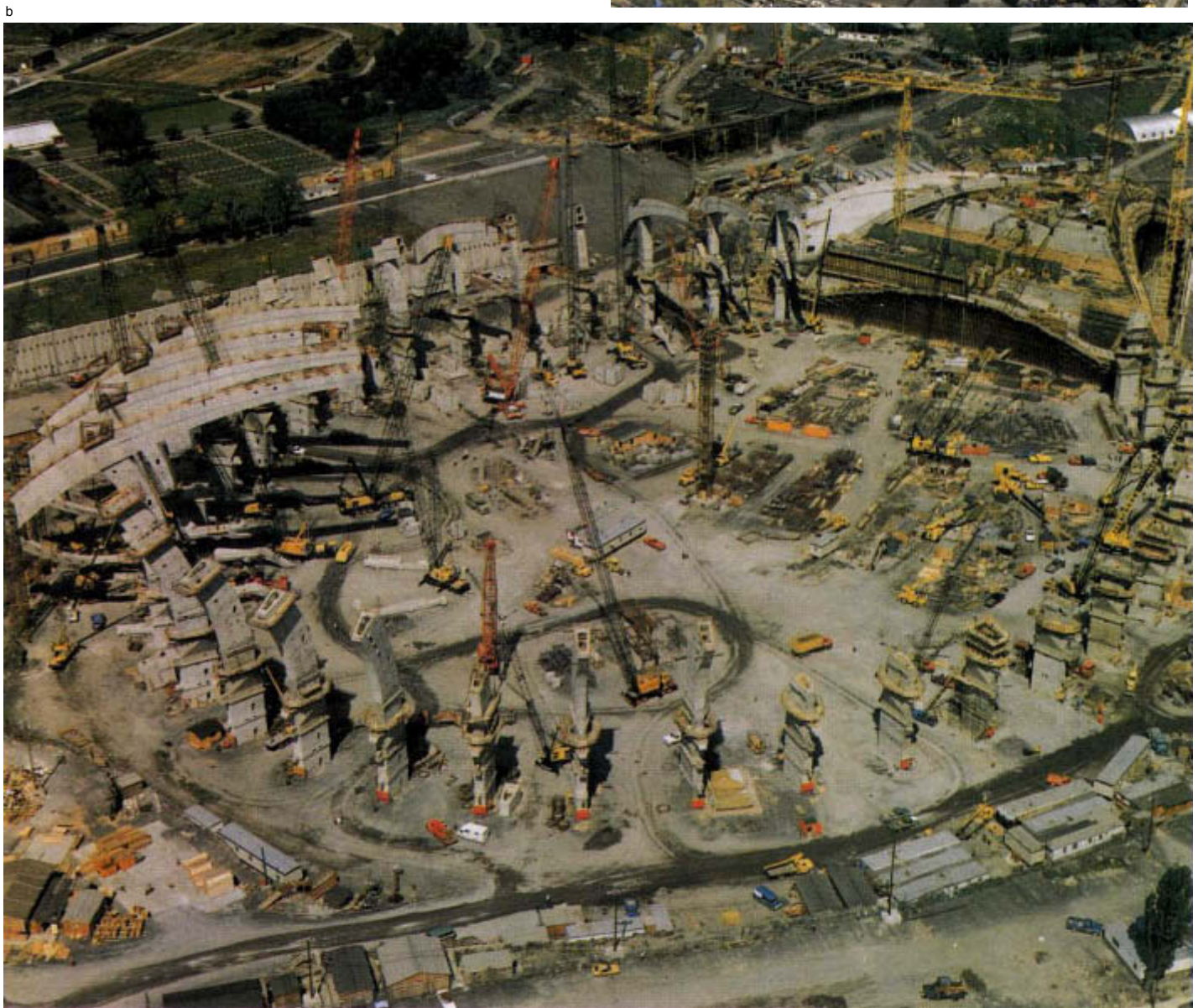
Stages of construction at the Olympic Park in July (a), August (b) and September (c) 1975.
