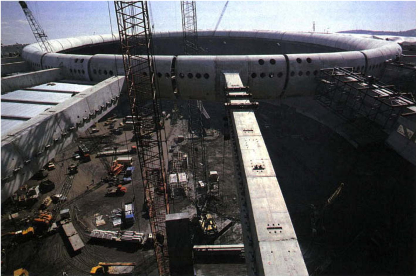
The final section of the technical ring is put into place on March 29, 1976.
