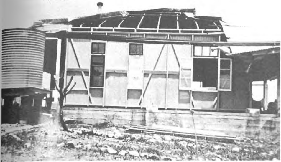
16. Cyclone damage at Channel Island leprosarium — Darwin March 1937. (Photos 14, 15, 16 reproduced by permission of Department of Territories and Local Government from originals held in Australian Archives, Canberra).
