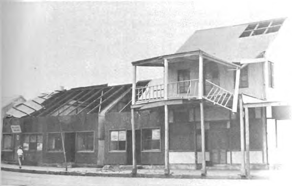
17. Cavenagh Street, Darwin March 1937 cyclone damage. (Bureau of Meteorology).
