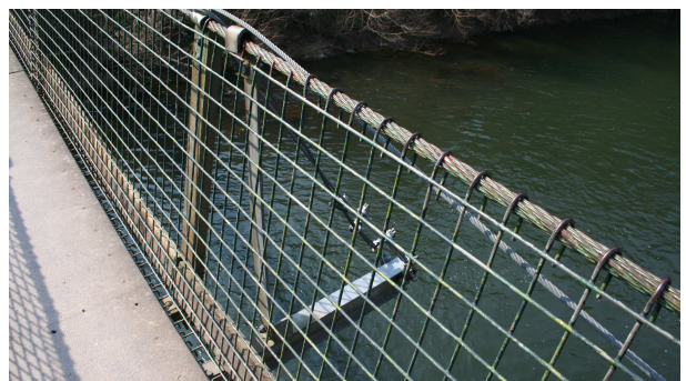
Figure 8: Attachment point for bracing cables
