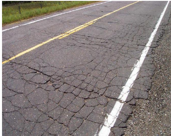
Figure 9. Severely Deteriorated Pavement Surface Condition
