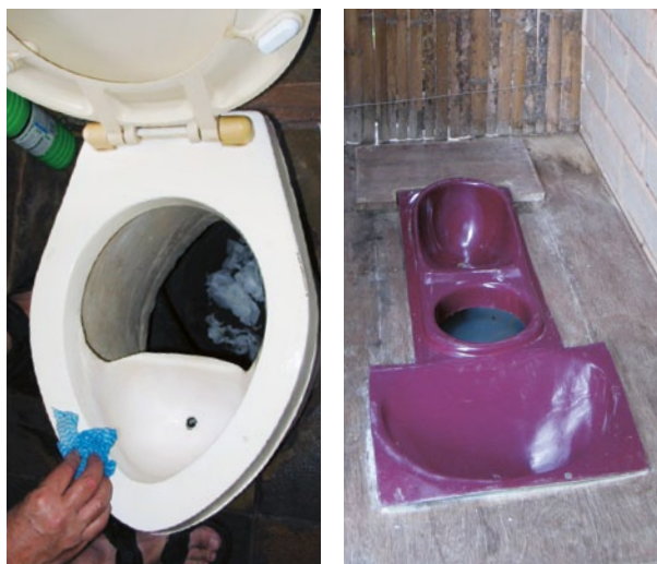
Figure 5. Left: Indoor UDDT (pedestal type) in Johannesburg, South Africa in the house of Richard Holden (source: E. v. Münch, 2006). Right: UDDT squatting pan in Bangalore, India, with three holes: the area in the front is for anal washing, middle is for faeces and back is for urine (source: D. Schäfer, 2008).
