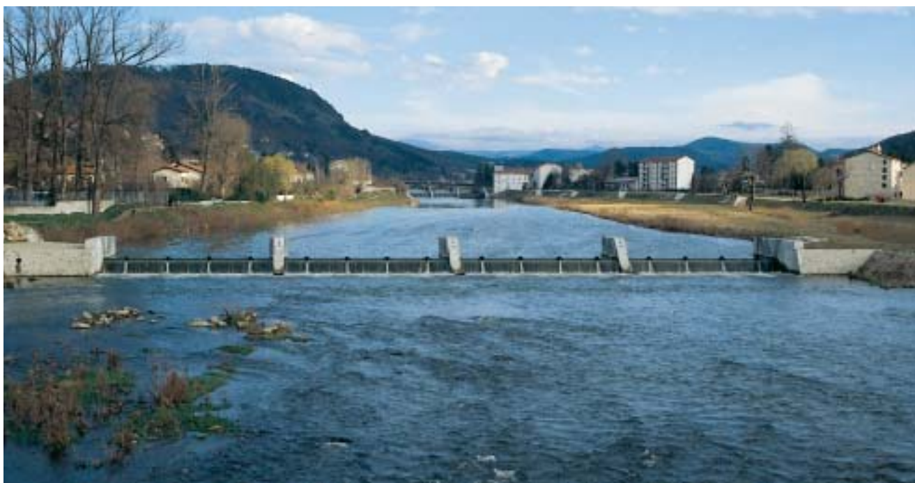
The first of three new removable sills installed on the Loire to restore the river's floodplain. WWF / SOS Loire Vivante
