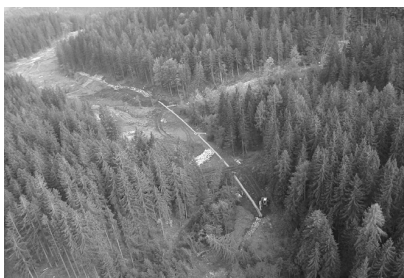
Fig. 2 The photo of the Macesnik Landslide in its upper part showing the execution of surface drainage works taken by R. Fazarinc in 2004
