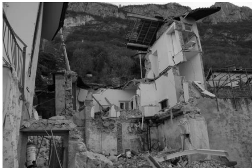
Fig. 1 Rockfall in the North of Italy.
