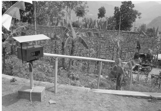
Fig. 1 Automatic extensometer installed at the upper part of houses at a dangerous zone.
