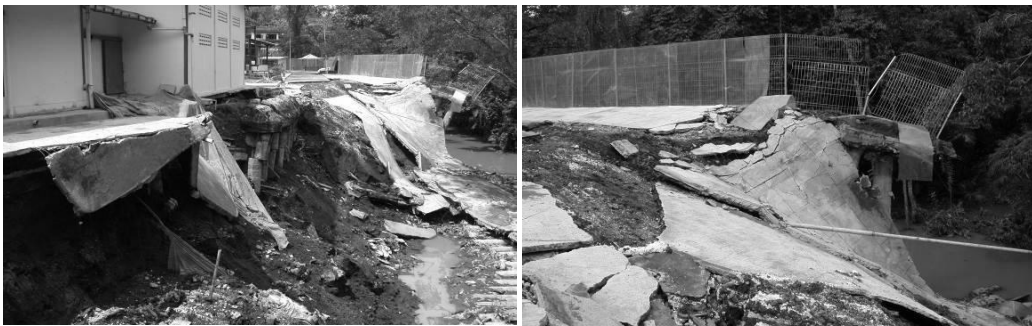
Fig. 1 The landslide threaten the factory building
