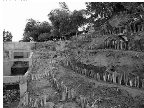
Fig. 4 The same slope now has improved drainage, and the slope has been planted in Vetiver grass.
