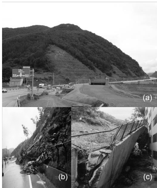
Fig. 2 Realities of cut slopes in Korea. (a) Steep and high cut-slopes in mountainous areas, (b) Cut-slope failure, (c) Retaining wall failure.
