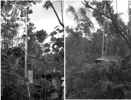
Fig. 7 Center pole (P2) was destroyed by landslide movement on December 30 th 2007.
