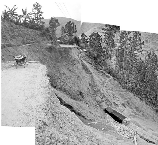
Fig. 4 Landslide on the B1 road at Section in Portland Parish, Jamaica
