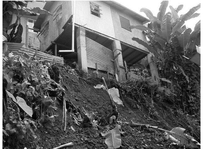
Figure 1. Example of a typical landslide in an unplanned community.
