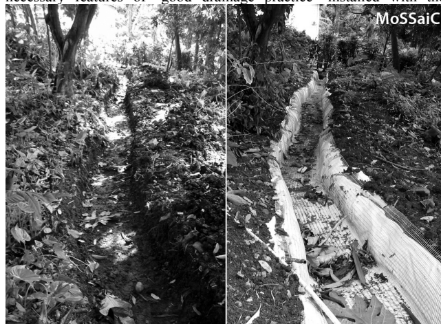
Figure 3. STAR TM drainage system installed by residents in St Lucia
