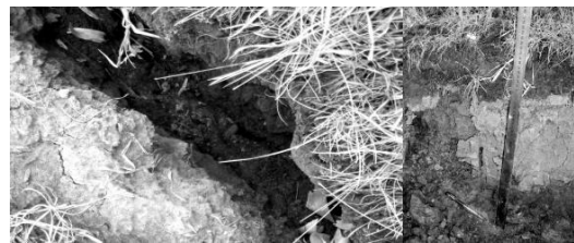
Fig. 1 Sandwich ice and freeze-thaw destabilization on the surface produced in the road cutting slopes of Jiamusi-Harbin section of Tong-San Highway
