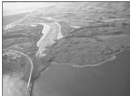
Fig. 3 Overview of central corridor cut to stabilize overall slope. Original road alignment to left in photo.
