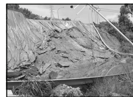
Fig. 7 Landslide incidence at Karambunai, Sabah recorded landslide risk of VHL3
