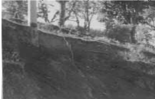
c. Electric pole at risk due to slide (Pyuthan district)
