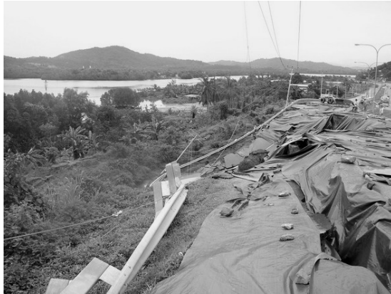
Figure 5. Road embankment failure buried a house at Bundu Village.
