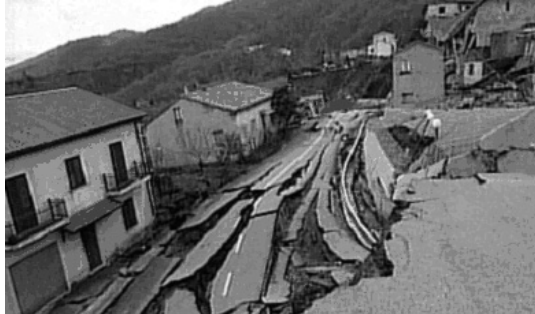
Fig. 2 The main road disrupted by the landslide.
