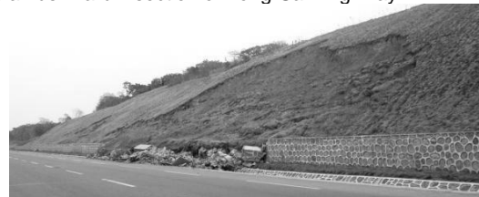
Fig. 2 Freeze-thaw destabilization of the road cutting slopes of Jiamusi-Harbin section of Tong-San Highway
