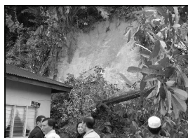
Fig. 9 Landslide incidence at Kampung Sungai Bukit Putih, Ulu Klang, Selangor recorded landslide risk of CL5
