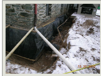
The project ran during the Winter months which increased the difficulty with sub-surface work.
