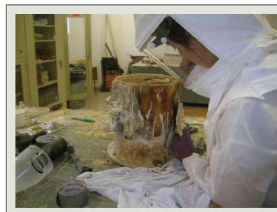
The existing columns ended the two wing walls separating the front and rear parlors. They were extremely deteriorated and lead based paint had to be removed.
