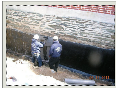
Several coatings were applied to the stone foundation to repel water from entering the buildings basement. A perimeter drainage pipe was also installed.
