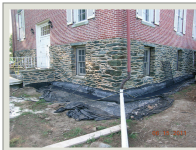
This shot was taken after the foundation wall has been coated with mastic to repel water.
