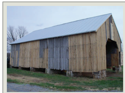
This Best Farm Corn Crib as seen after the extensive stabilization work completed by the HPTC Carpentry Team.
