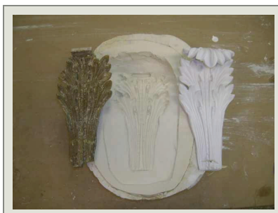
At the column capitals new acanthus leaves were made from castings produced from the originals.
