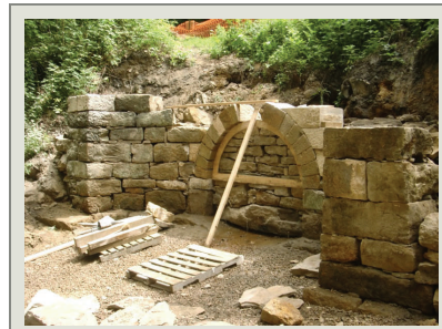
Field engineering reduces costs. The HPTC Exhibit Specialist directing the job devised a stabilization approach that eliminated the need to repair the culvert tunnel.
