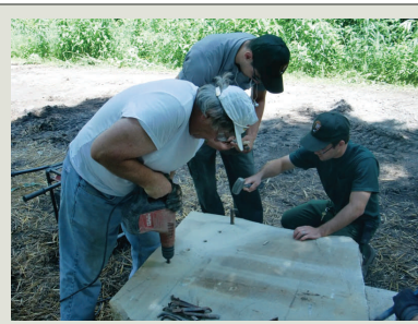
Several field training sessions for park staff were incorporated into this project. Here Park trainees lay-out and make stone block cuts.
