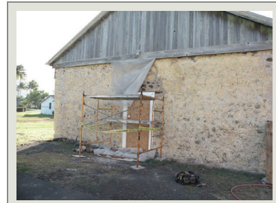
Similar repairs were also required at the former door opening that had also been blocked up when the building was a jail. New windows and doors were fabricated.
