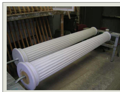
The restored capitals will be re-joined with the repaired fluted wood columns when the columns are reinstalled in the Thomas House sometime early in FY12.
