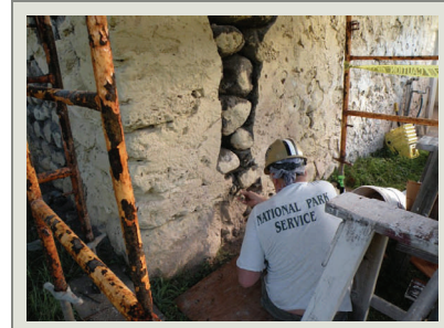
The project objective was to repair the exterior masonry and apply a skim coat of stucco. The building now serves as the park's Ranger Station.
