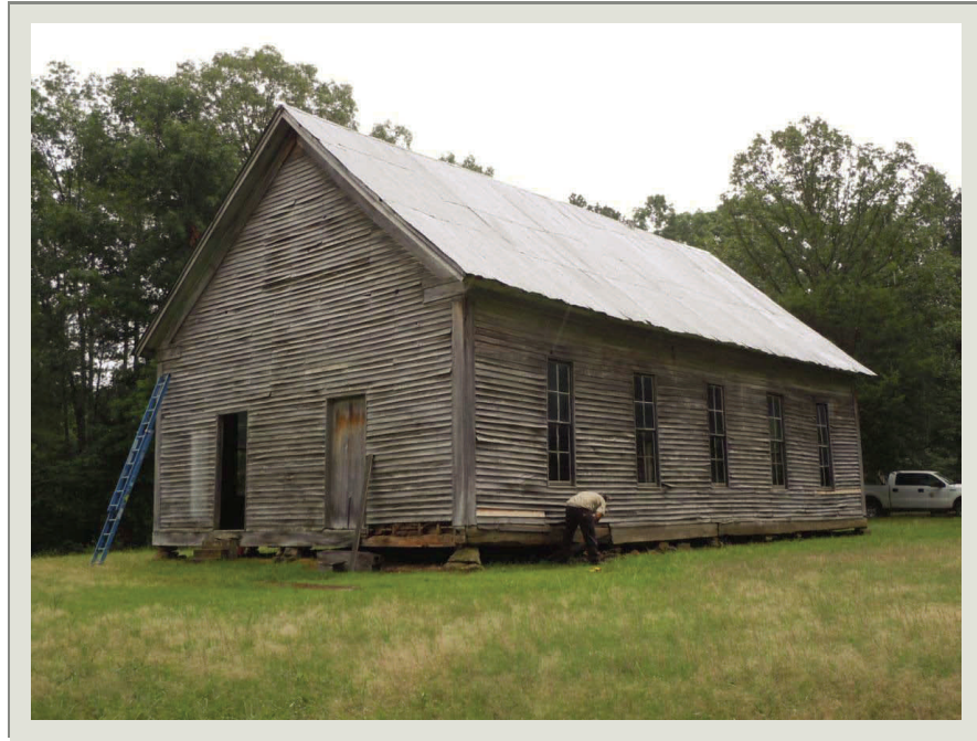
Tennessee National Wildlife Refuge—Mt Zion Church Historic Structure Assessment Report. This report was completed in FY11.
