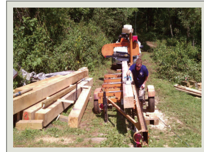
Carpentry Team members Dean Harper and Nate Ramsier maneuver a timber onto the leveled HPTC sawmill.
