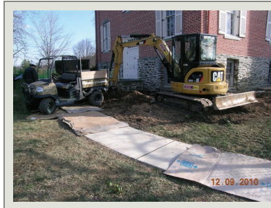
This project was designed under a contract managed by the HPTC Project management team. The project goal was to improve foundation drainage.
