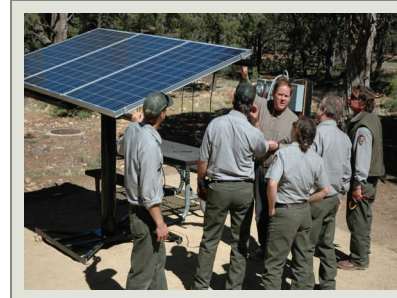
Two 2011 NPS Photovoltaics classes funded by the Maintenance Career Academy at the Grand Canyon taught staff installation and troubleshooting of solar panel systems.
