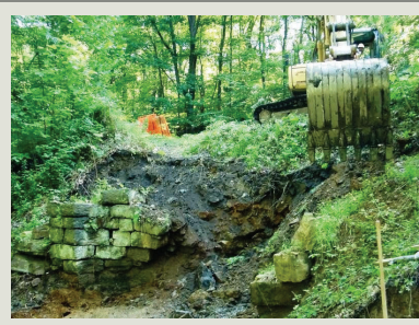
The collapsed headwall at Culvert #299 threatened the path used by park visitors travelling along the portage trace above the culvert.
