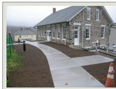
This view shows the main entrance to the Anthony Library with the landscaping work recently completed. The Anthony Library contracts are due to be entirely completed by the end of December 2011.
