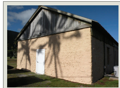
This Final Inspection photograph shows the stone façade of the Old Church after the completion of the HPTC project work.
