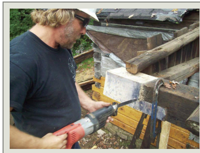
HPTC Maintenance Mechanic Paul Jensen uses a reciprocating saw to tighten the half-lap repair on the porch's lower plate timber.
