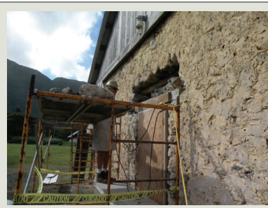
HPTC Masons made required stone repairs at the former window openings that had been filled in with concrete blocks during the jail era.
