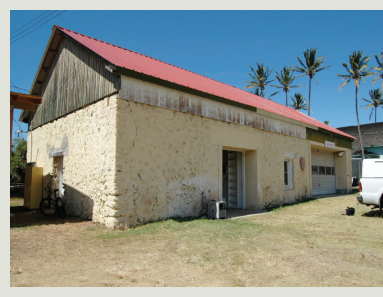
This "before" photo shows the 1853 Old Stone Church as it appeared before rehabilitation. The building had also previously served as a jail and a warehouse and had been extensively altered.
