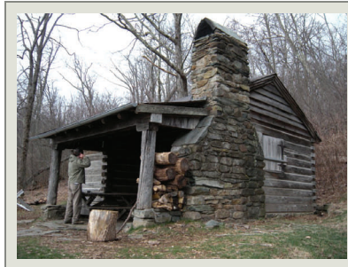
The Pocosin Cabin Log Cabin before HPTC work. This backwoods cabin was built c1933 and serves hikers travelling along the Appalachian Trail in the park.
