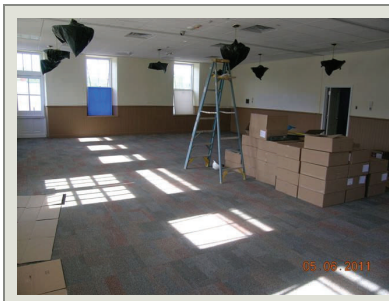
The main room of the former library has been converted into meeting and conference space for use by the HFC.
