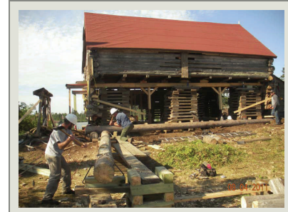
The first task completed by the HPTC team was to safely jack the building back into its proper alignment.
