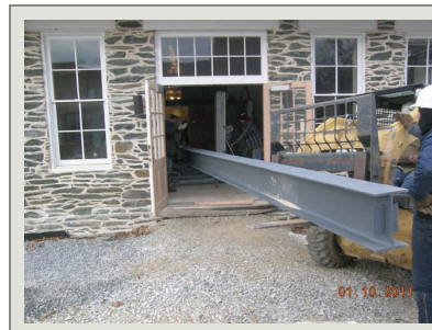
The interior repairs have been completed by contractor. The entire interior volume of the Anthony Library has been extensively rehabilitated.
