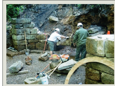
The stabilization objective of this project was to halt the ongoing erosion that threatened the trace walkway.
