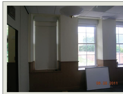
Character defining historic interior fabric, such as the wood wainscoting, seen in this photo, has been carefully restored.
