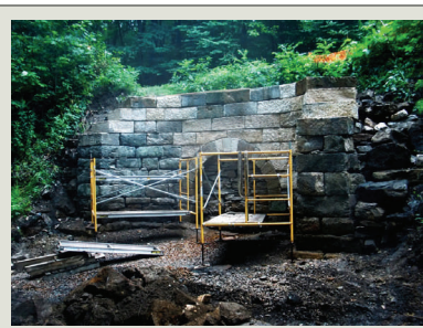
The stabilized Culvert #299 nears completion. New cut replacement stone blocks were required necessary to complete the rebuilding of the headwall. The entrance to the tunnel is delineated by rough, coursed field stone.
