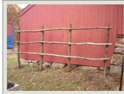
The HPTC reconstructed the Barn Trellis based upon historic photographs. The HPTC then prepared drawings for approval prior to construction.
