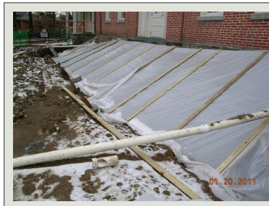
The contractor was forced to protect the work area from the severe winter weather. The project also included repairs to the gutters and downspouts.
