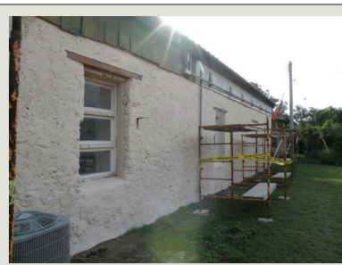
A wash coat was applied to the masonry exterior after the repairs were completed. Reconstructed wood window sash were installed in the historic window openings.
