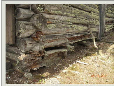
The deteriorated sill logs of this 19th century rustic log tourist lodge were the root cause of the structural failure of the building.
