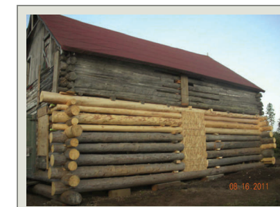
The opposite elevation of the Johns Lodge was stabilized using replacement in-kind logs. More logs must be harvested and dressed to finish this elevation.
