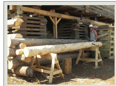
Replacement logs are dressed using hand tools to match the deteriorated sill logs removed by the team. Contracting for this type work at remote Isle Royale would be problematic.
