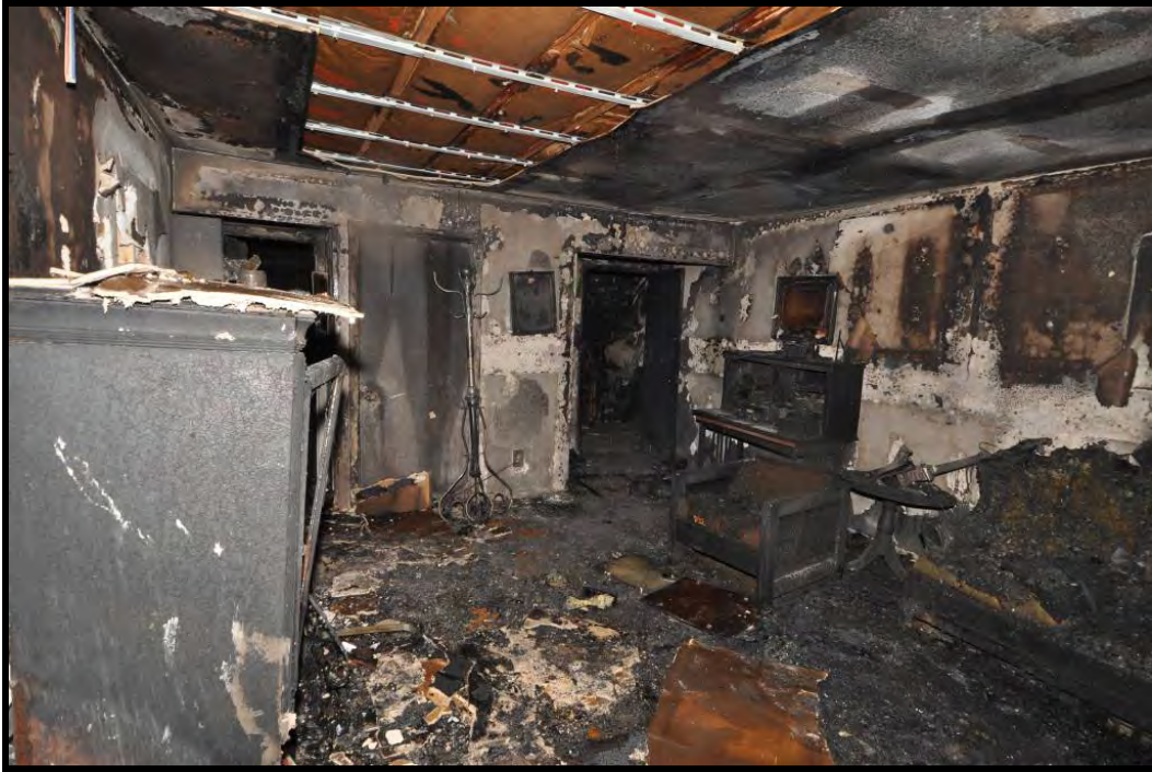
Figure 60. Photo of living room that experienced flashover in apartment A2. The hollow core bedroom door is located in the small hallway at the upper left of this photo.
