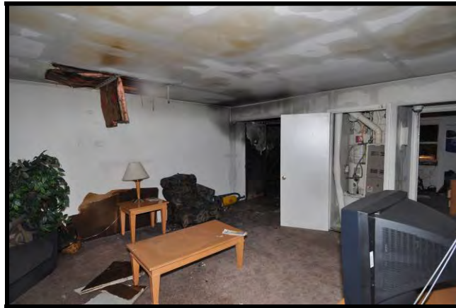
Figure 52. Photo of damage to apartment A1. Door was closed for majority of fire.
