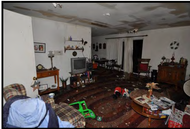
Figure 49. Damage to apartment T1. Door was closed for majority of the fire.
