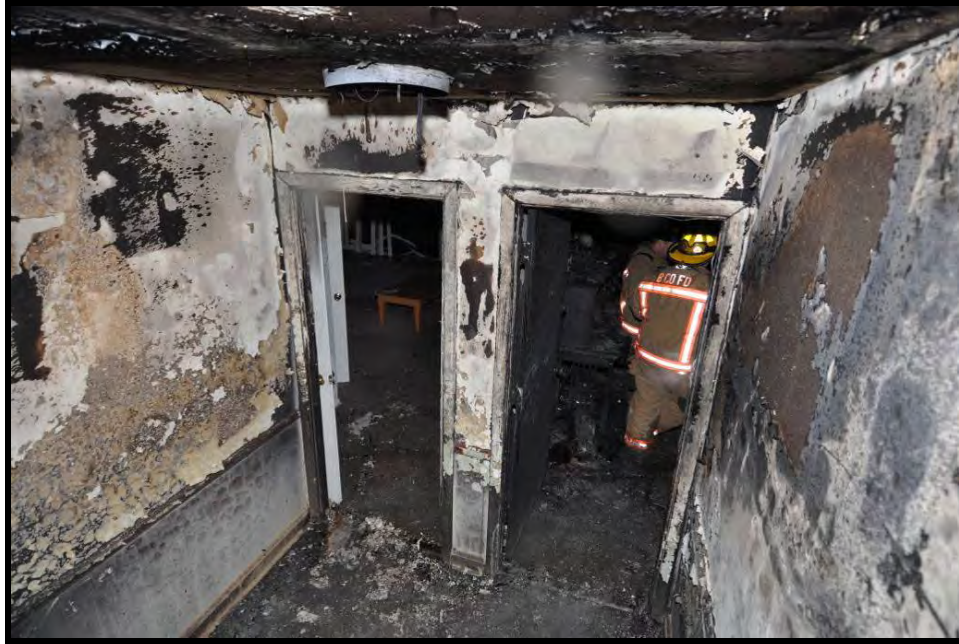
Figure 51. Photo of second floor stairwell landing and apartments A1 (left) and A2 (right).
