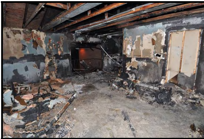
Figure 56. Damage to apartment B2 (post overhaul). Door was left opened by search crews.
