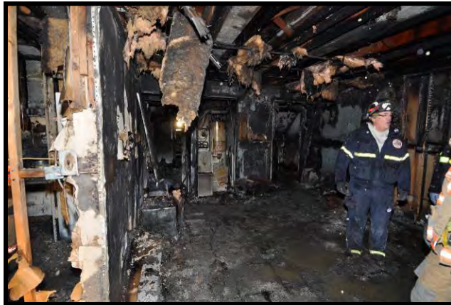
Figure 50. Damage to apartment T2 (post overhaul). Door was opened by occupant after discovering the fire.
