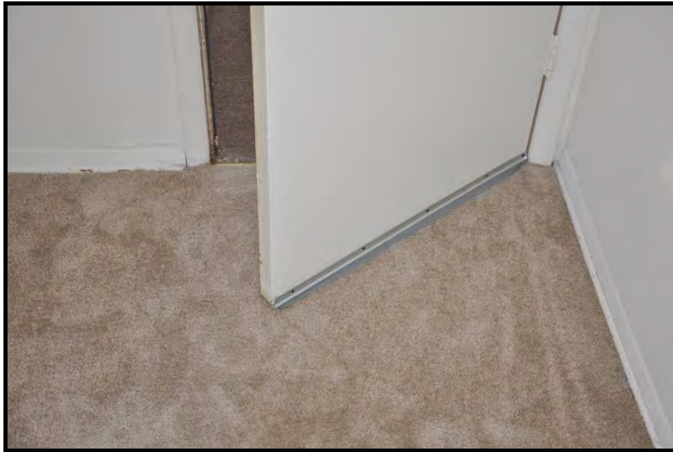
Figure 24. Close view of base of the door impacting the carpet, preventing the door from self closing.
