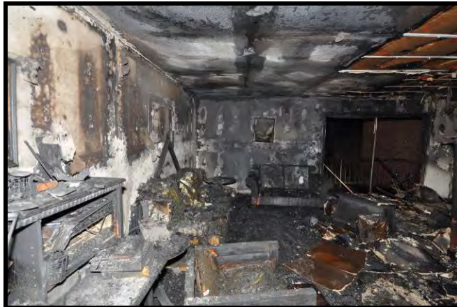
Figure 53. Photo of damage to apartment A2. Door was left opened by search crews.
