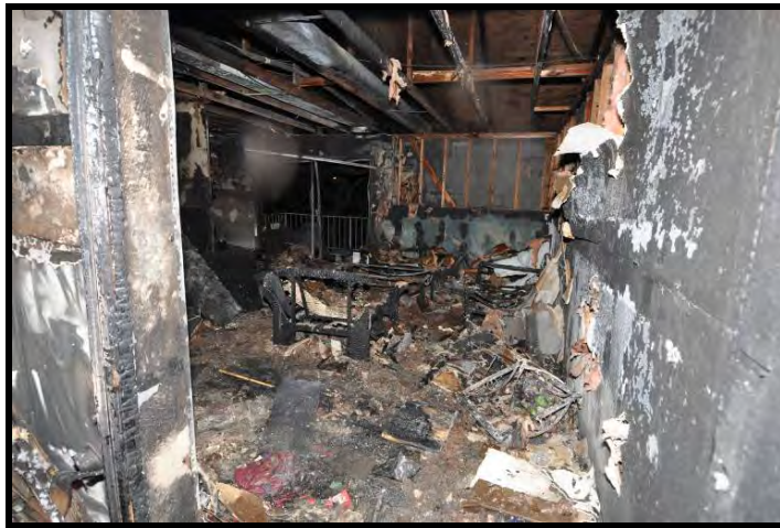
Figure 55. Damage to apartment B1 (post overhaul). Door was left opened by search crews.
