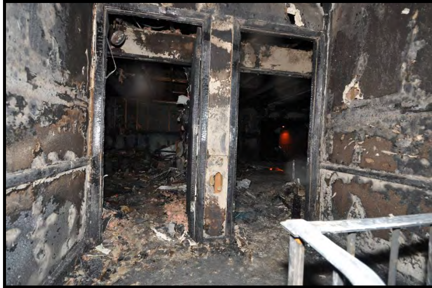
Figure 54. View of the third floor landing looking in at apartments B1 (left) and B2 (right).
