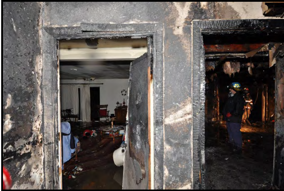
Figure 48. Terrace level stairwell landing looking into T1 (left) and T2 (right) apartments.
