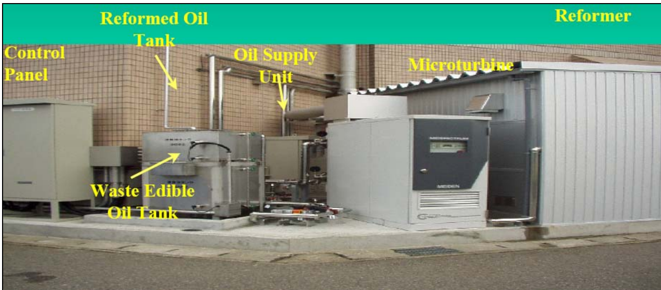
View of the system - Project Site: A Public Hospital in Ishikawa Prefecture
