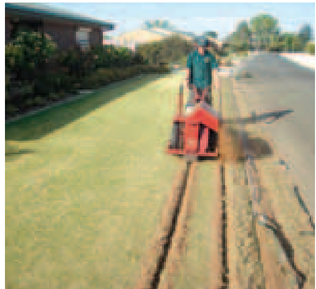
Irrigation installation by Berri Native Plants, Berri, South Australia, using the TRENCH'N edge Trencher. Photo supplied by Andrew Walladge, Berri Native Plants
