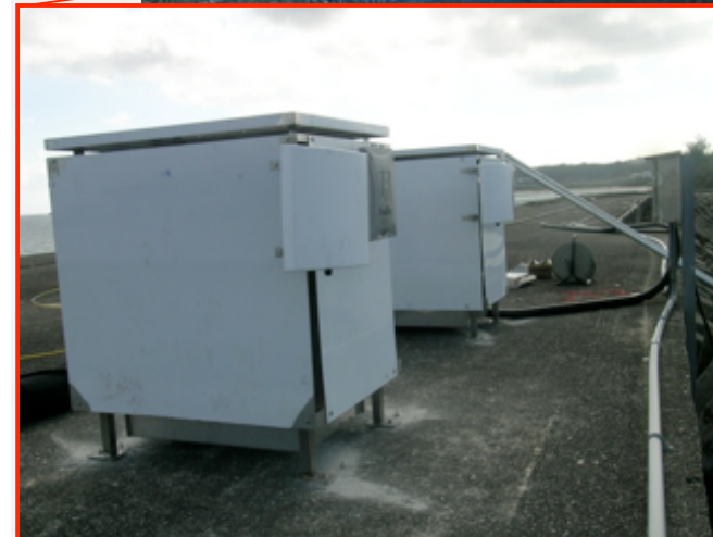
▲ Nuclear Power Plant 3
