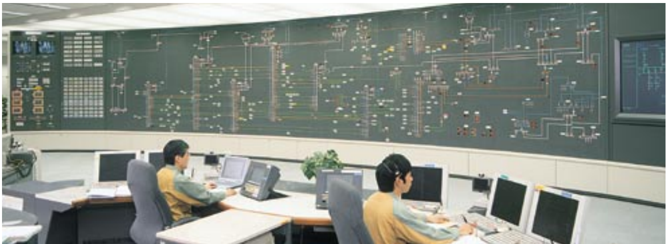
▲ Load-Dispatching Control Center
