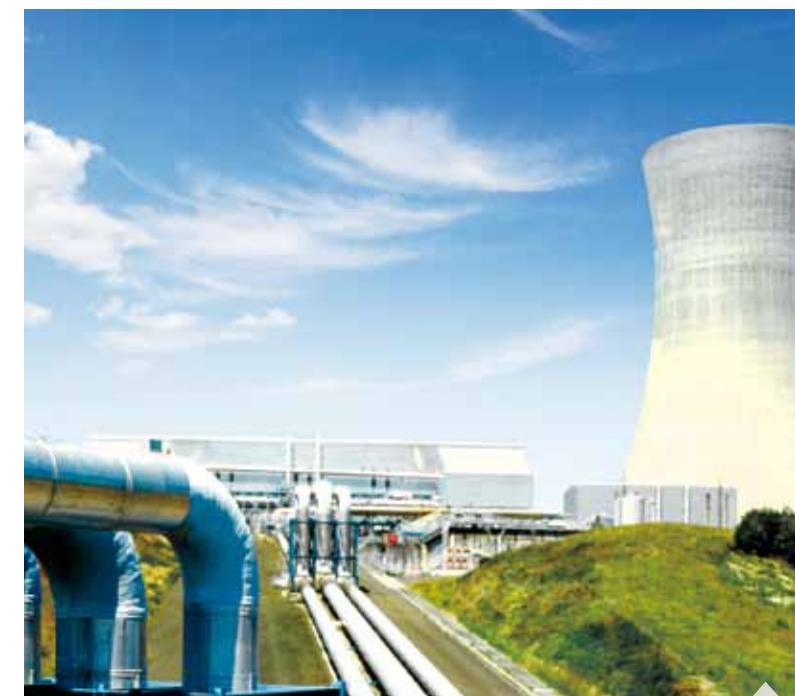
Fuel delivery pipeline
