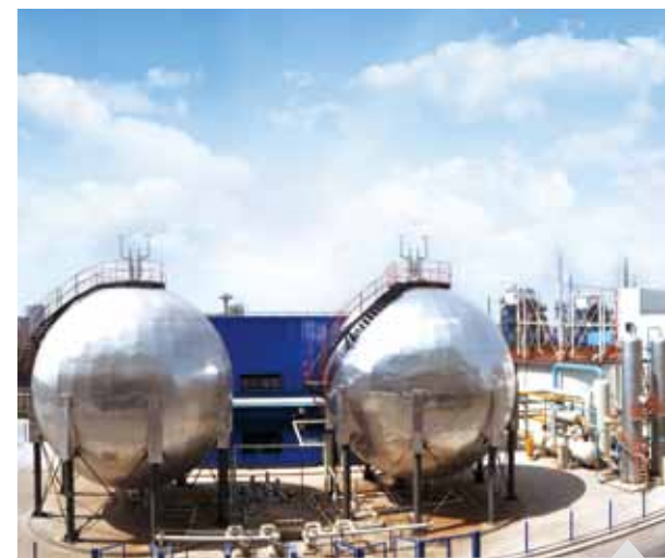
CO 2 capture devices in the Shidongkou Power Plant II
