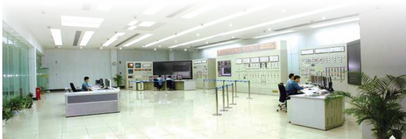
Modern power plant control centre
