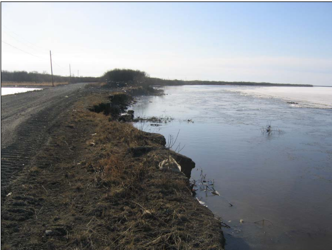
Erosion at the community of Emmonak
