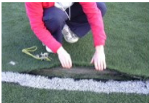
Poorly made joints can create hazards to players. A comprehensive programme of quality monitoring helps eliminate poor workmanship
