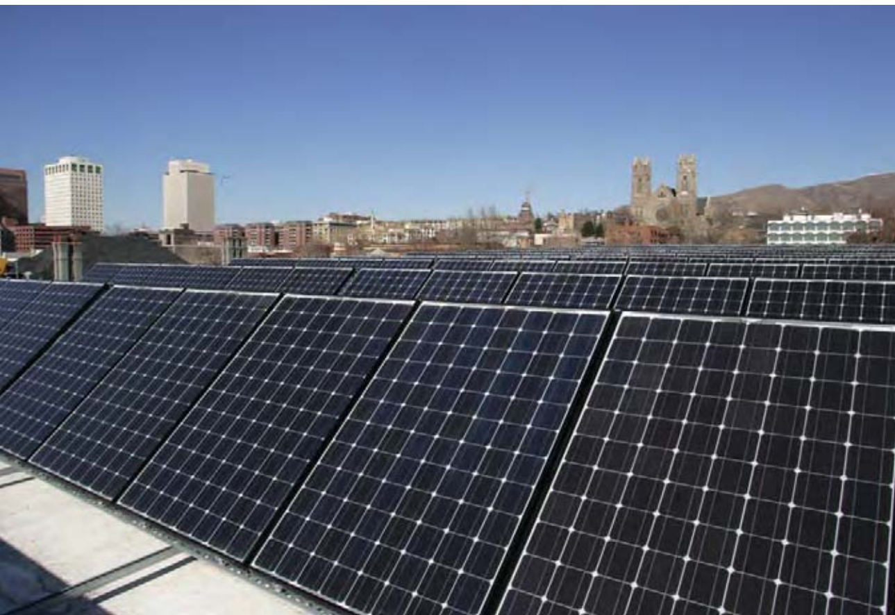
A 25-kW solar PV system provides power to the county-owned Clarke Planetarium in downtown Salt Lake City. (SLC/PIX18364)
