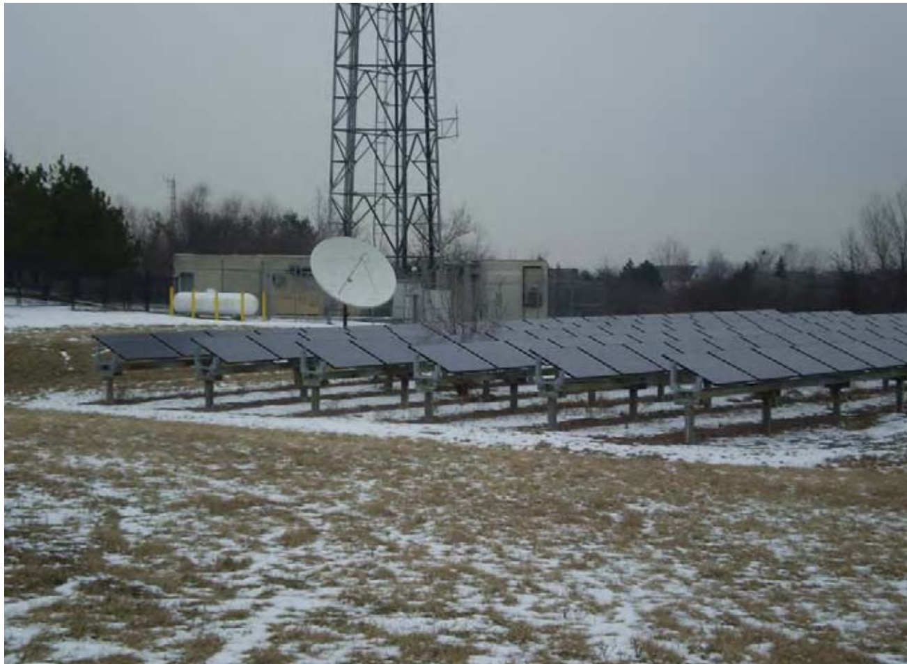
The 100 kW ground-mounted PV system is co-located with an electrical substation in Ann Arbor, Michigan. (Vipin Gupta/PIX179326)
