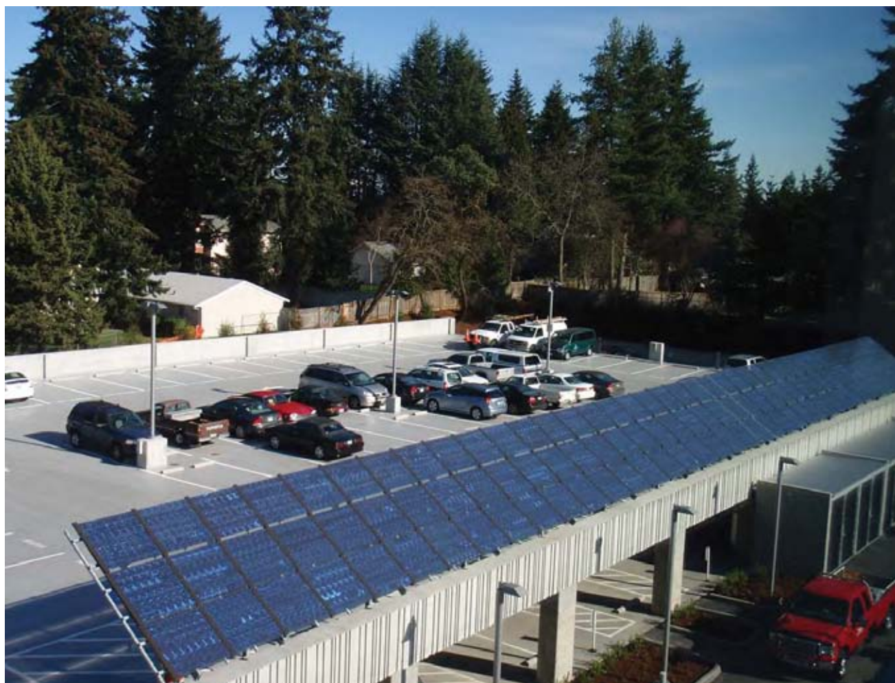
The City of Shoreline, Washington, installed a 20.2 kW solar electric system on top of the City Hall parking garage. The system uses Washington-made solar modules from Marysville-based Silicon Energy. (City of Seattle/PIX18074)
