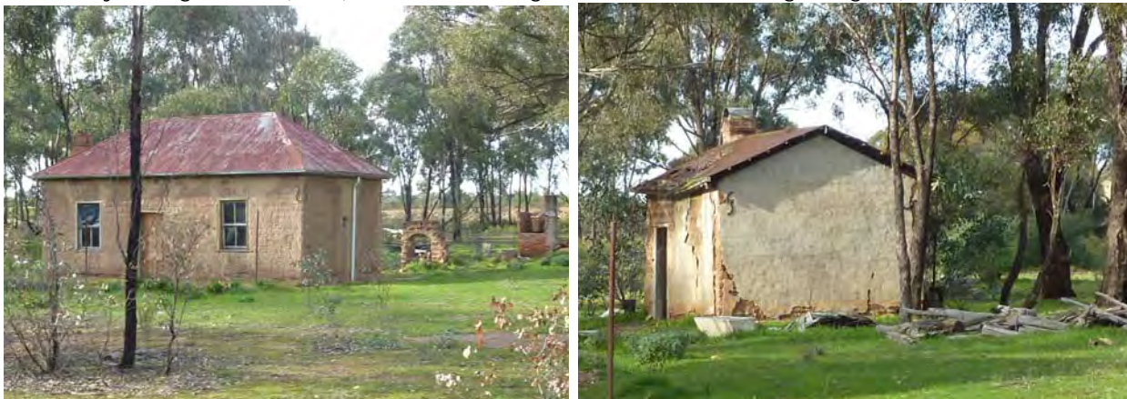
Left: West and south elevation of the cottage, note ruins of former kitchen at rear. Right: The outbuilding as viewed from Caldow Road. Note poor condition of the roof and render.
