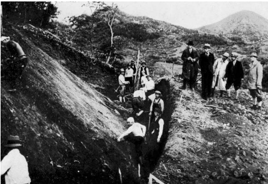
Mr. M. Zentzytzki (extreme right) who was invited to Japan to construct the bobsleigh course, supervising the construction.
