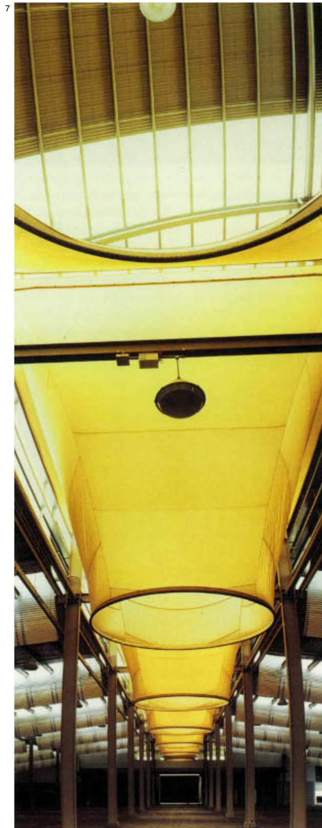
7. Ventilation ducts in the Showground draw hot air out of the Pavilions, creating a natural ventilation in line with the Sydney 2000 commitment to environmental engineering
