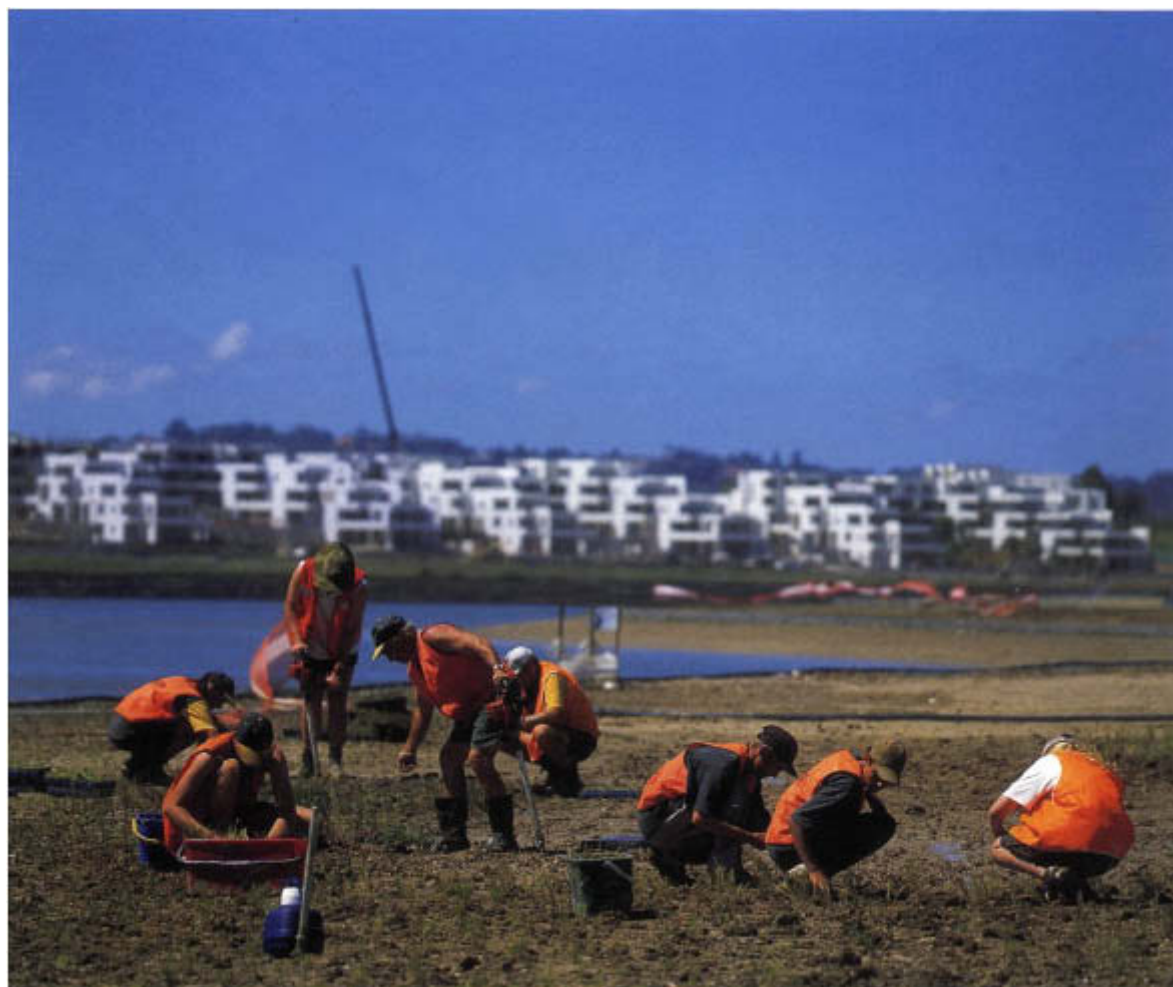
4. Workers near Newington plant trees after the extensive remediation exercise at Homebush
