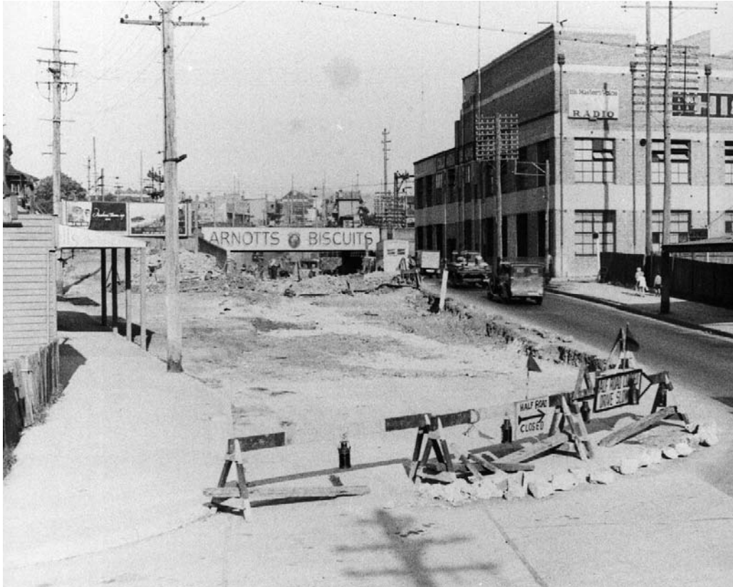
Figure 11 Maintenance, October 1938. Upgrading roads was a constant chore as seen on Parramatta Road near the Homebush underpass. Source: GPO I, 32541
