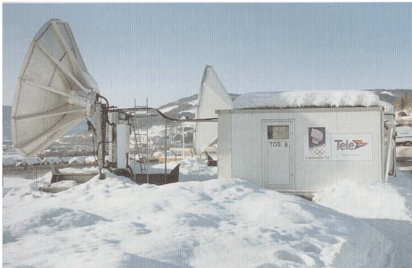
C-band containers with antennas of 4.6 m diameter at the IBC/Satellite site
