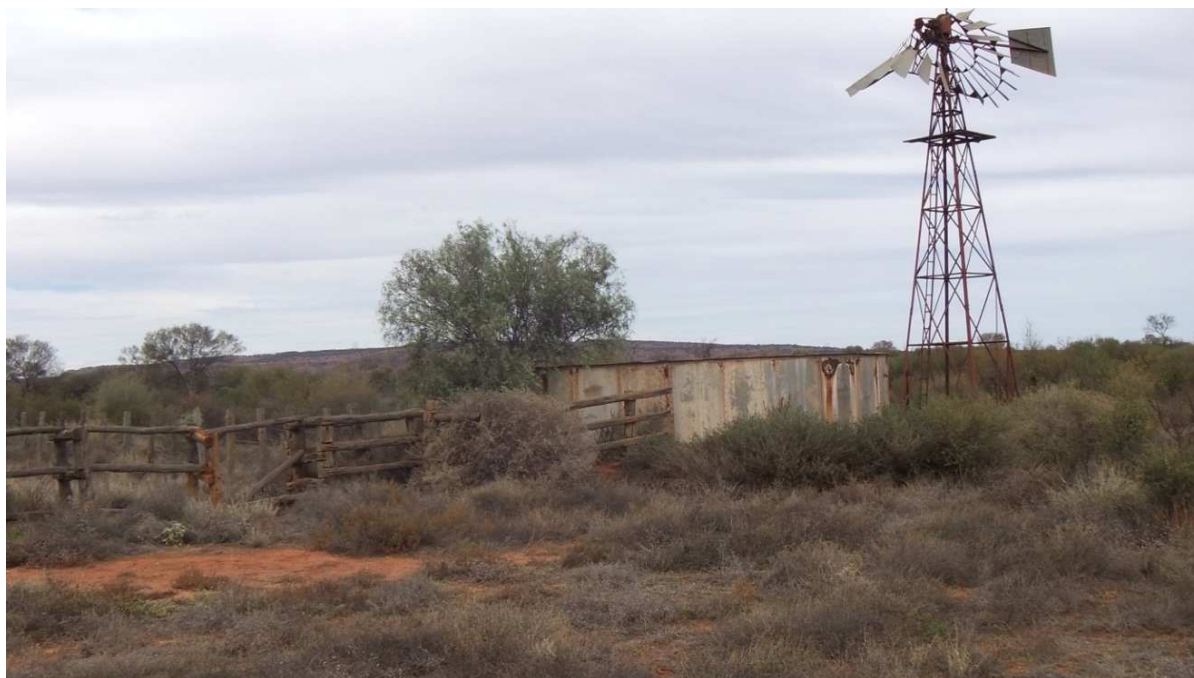
Figure 11: Davies' Bore – the windmill, water storage tank and timber fencing which will need to be replaced.
