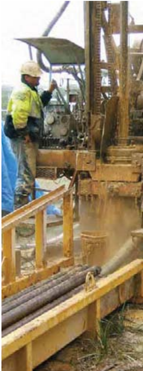
Upper Nepean groundwater investigations. A test bore being drilled deep into the sandstone to determine likely pumping rates.
