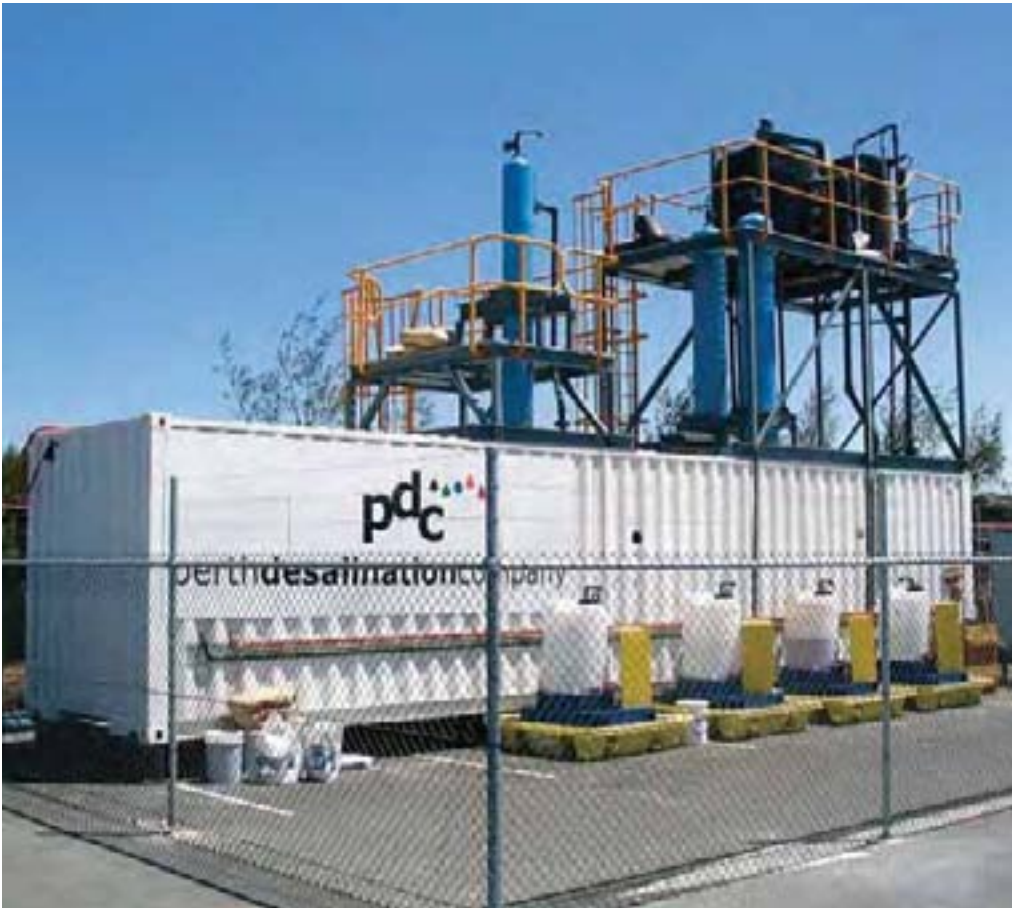
Example of desalination pilot plant in Perth
