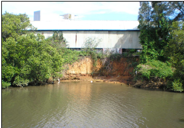
Bank Erosion – Upper Estuary (28/11/2007)
