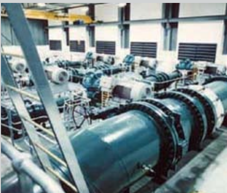
Belmont Pump Station, Perth
