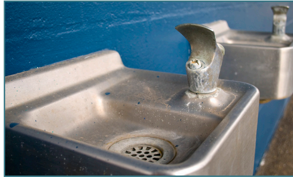
Lime build-up on mouthpiece and protective guard of drinking fountain.
