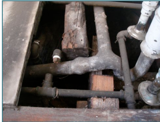
Example of lead pipes in a plumbing system.
