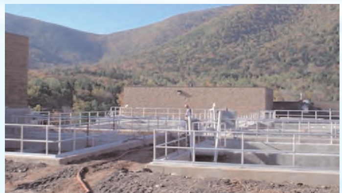
Hunter WWTP, Hunter, NY
