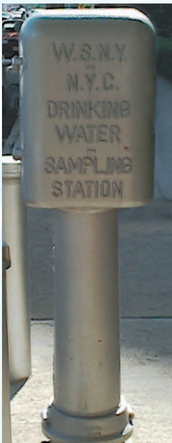
Drinking Water Supply Sampling Station
