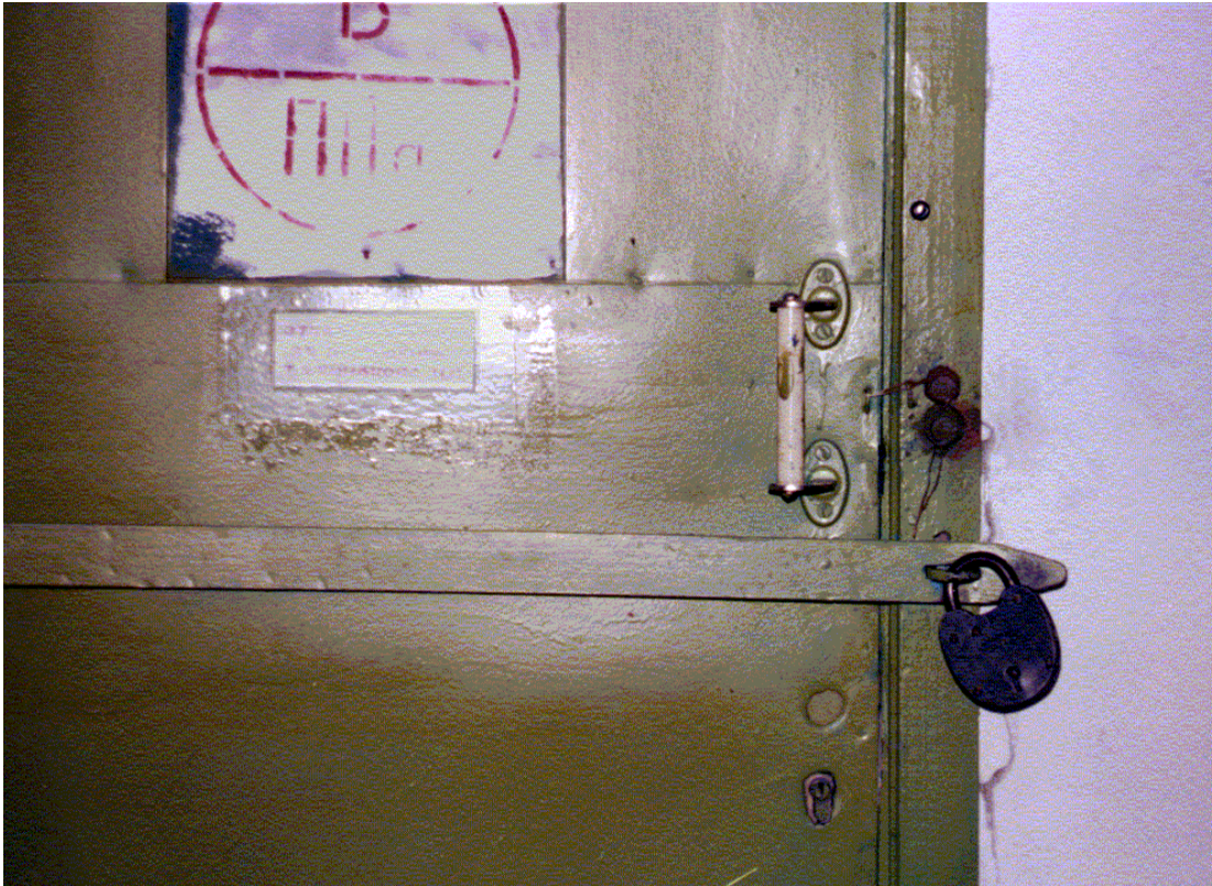
Figure 2.4: Ineffective Seal and Easily-Cut Padlock on Nuclear Material Door
