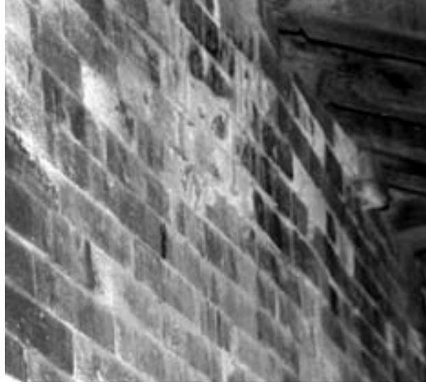
Fig. 89. Salt crystal on wall surface.
