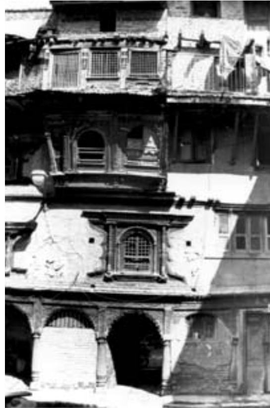
Fig. 55. Damage of carved elements.
