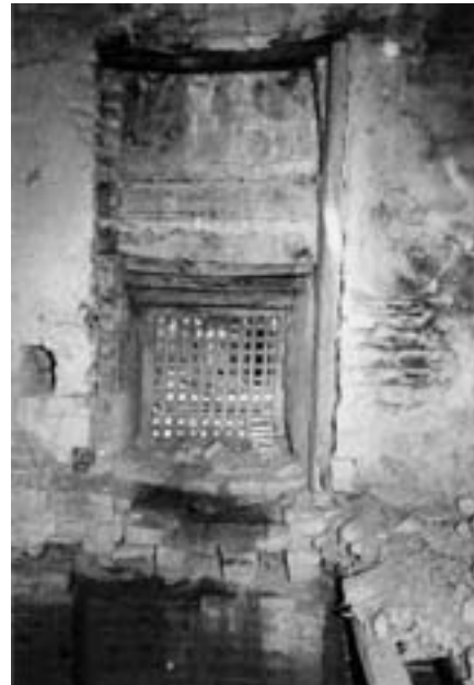
Fig. 43. Deterioration of timber elements from damp.
