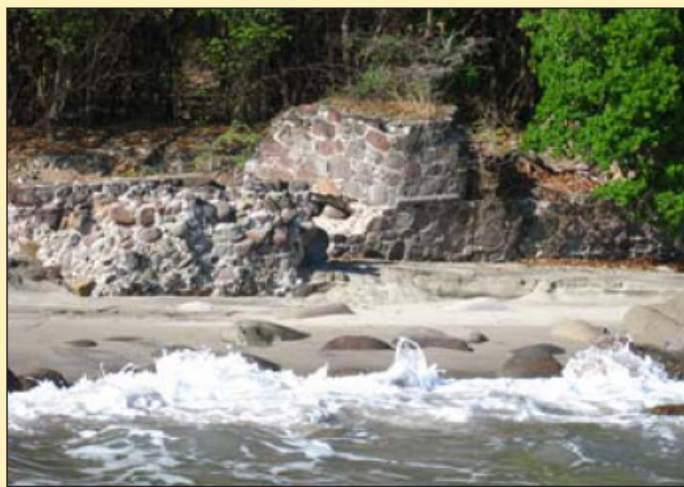
The Waterfort (or Fort Amsterdam), Statia's second oldest building, is in urgent need of repair
