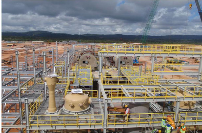
Figure 22. Cracking or Rotary Kiln at Lynas Advanced Materials Plant (LAMP) Rare earths refinery under construction by Lynas Corporation at the Gebeng Industrial Zone, Pahang, Malaysia. Source: Lynas Corporation.
