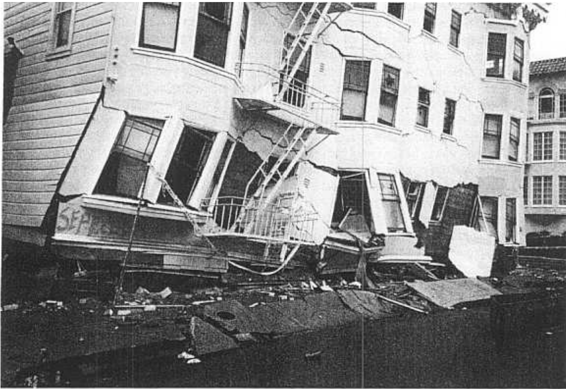
Figure 4.3 Buildings that failed in the San Francisco Marina District typically had structural vulnerabilities and were also built on soft-soil deposits.
