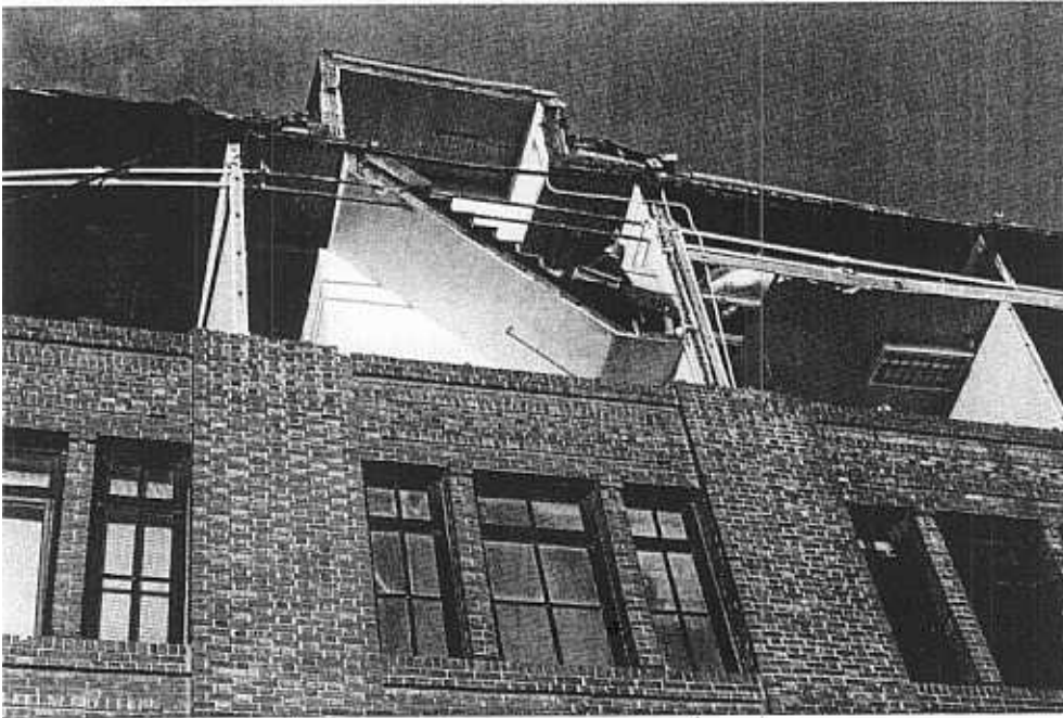
Figure 4.1 Unreinforced masonry building on 6th Street in the South of Market District of San Francisco that suffered major damage during the earthquake
