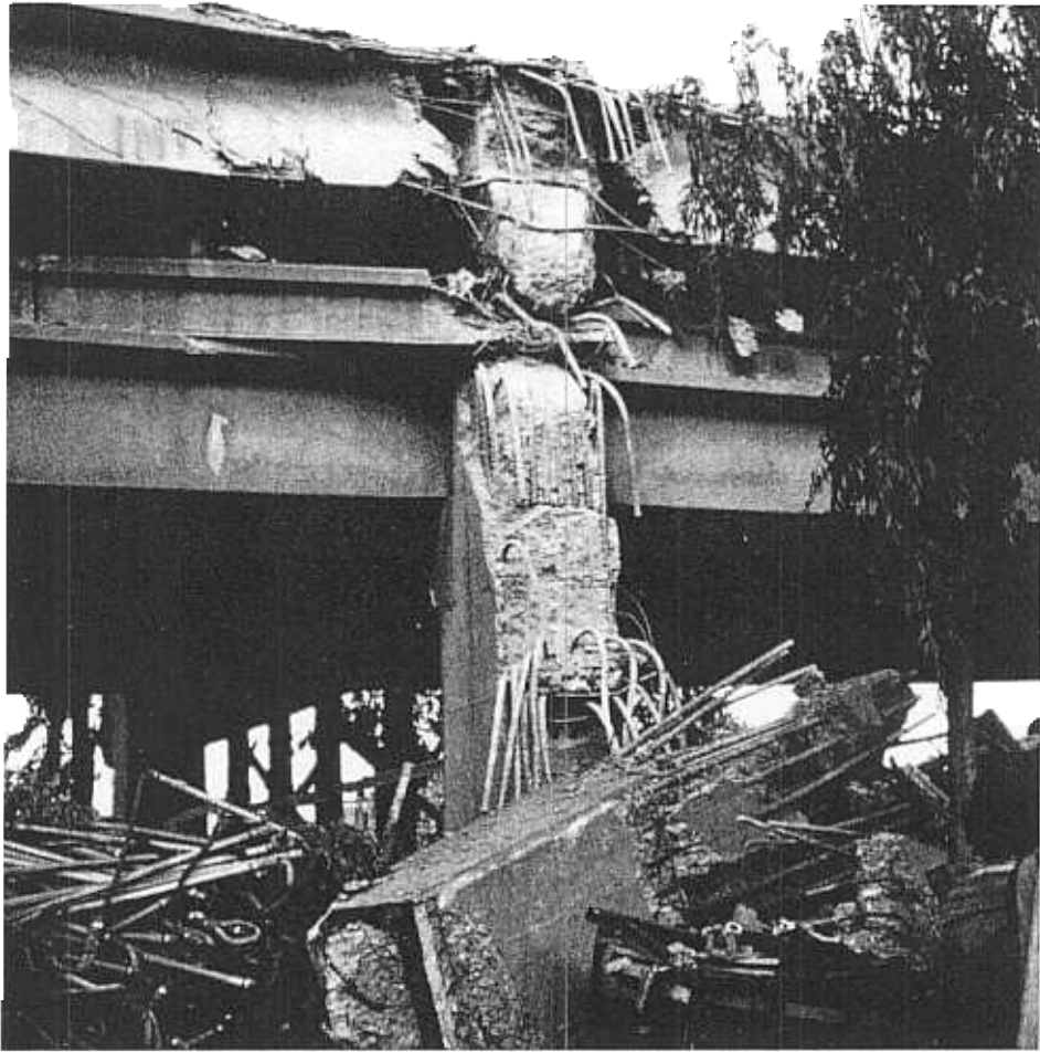
Figure 5.1 The greatest damage from the earthquake occurred to older structures on poor ground, such as the I-880 Cypress Street Viaduct.
