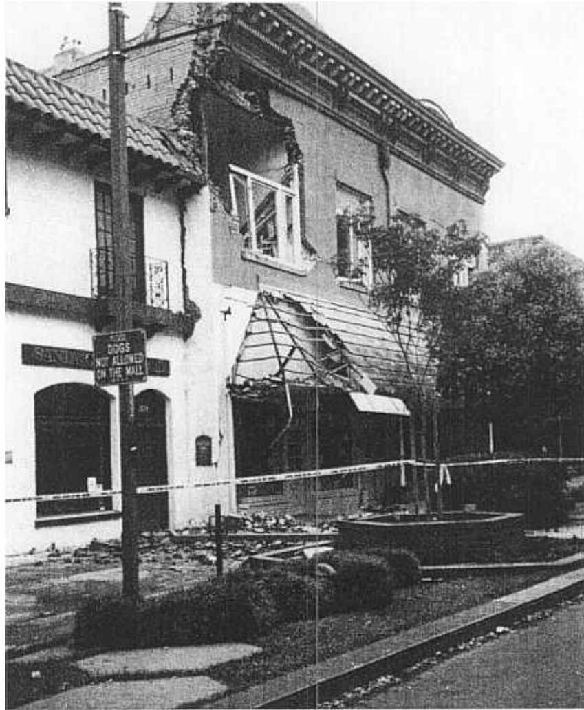
Figure 6.1 Although many of the structures on the Pacific Garden Mall in Santa Cruz were attractively and expensively rehabilitated, the improvements did not include appreciable strengthening and many were lost.
