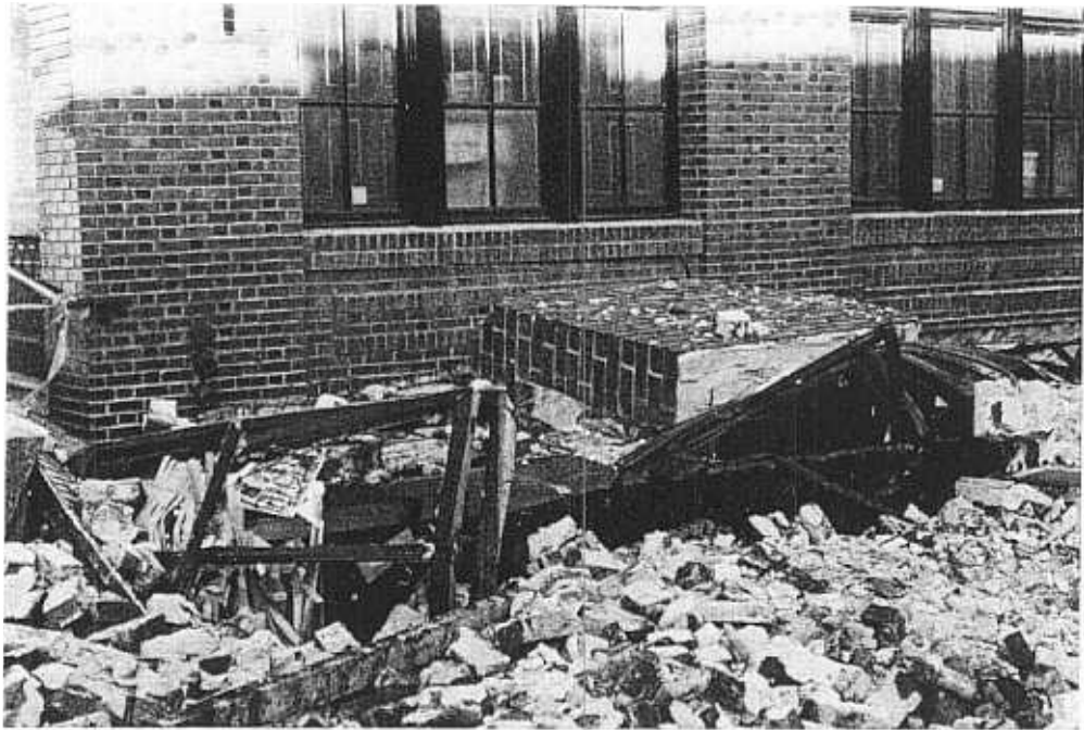
Figure 4.2 A portion of the unreinforced masonry wall that fell from a building on 6th Street in the South of Market District of San Francisco
