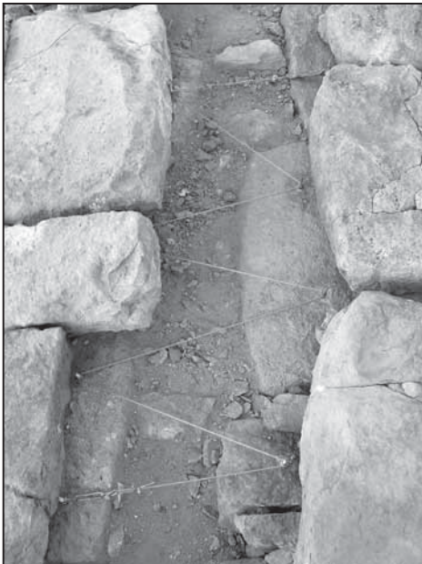
Fig. 11: Interior view of northwestern wall of Terrace Building 2, showing steel cable used to tie the two faces of the wall together
