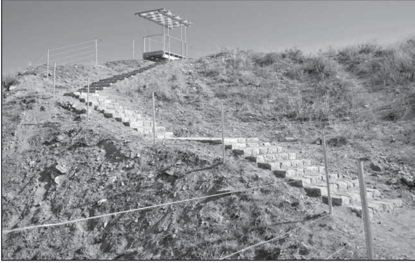
Fig. 14: Viewing platform on visitors' path at northeast, with newly installed stone staircase and metal fencing.
