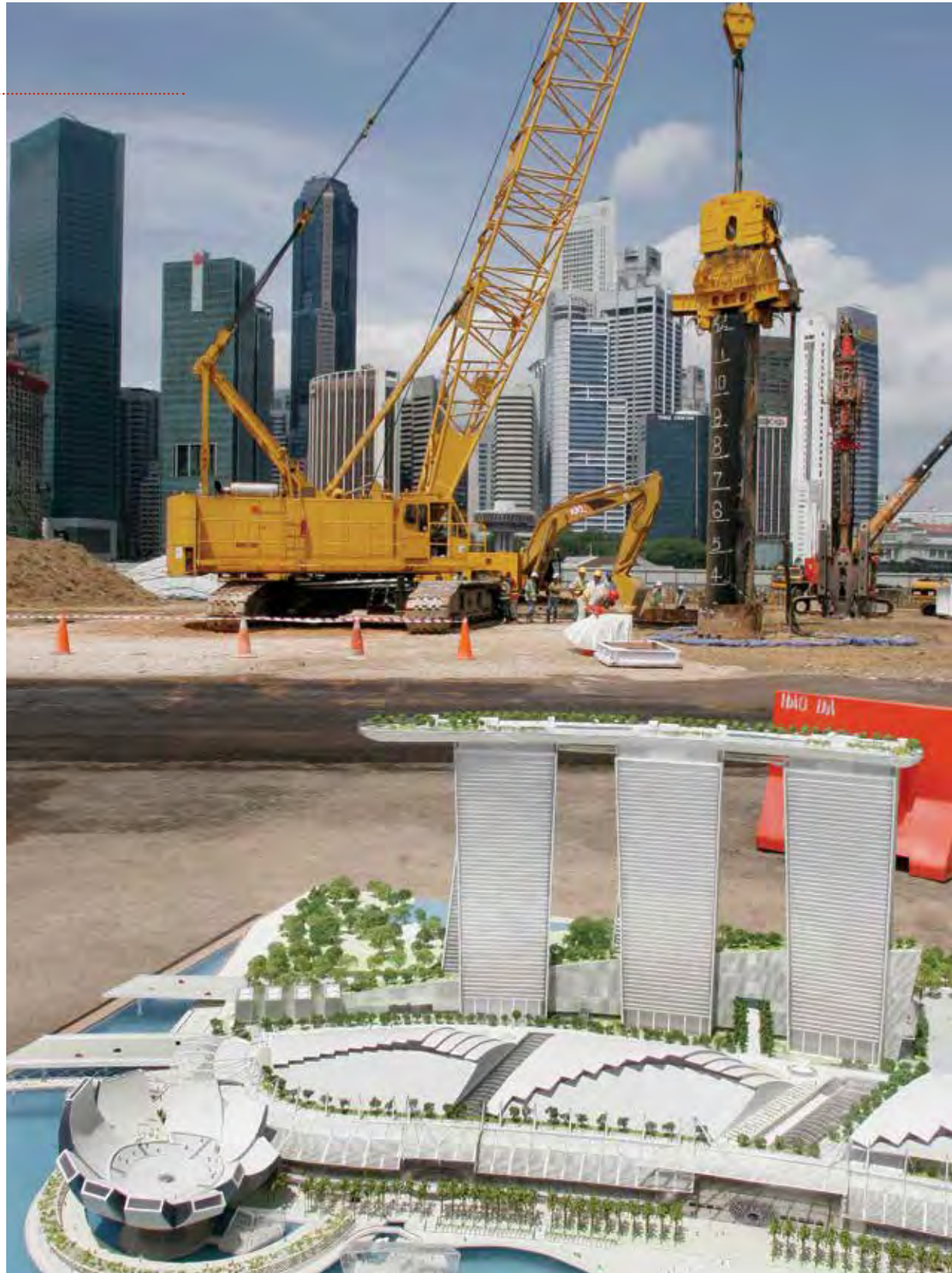
Work starts at a Singapore resort, with the city in background and a model of the Marina Bay Sands in foreground.
