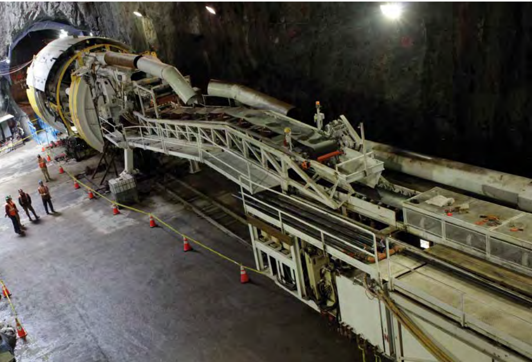
Digging into Manhattan's bedrock for the new Second Avenue Subway, on which Peter Chamley served as chief engineer.
