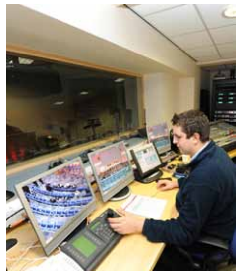
A control room in the lecture theatre
