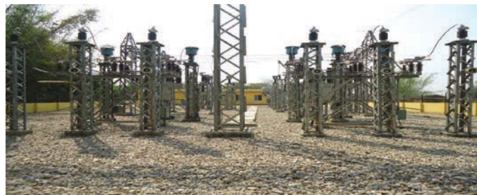
Completed Dhulabari 33/11 kV, 6/8 MVA Substation
