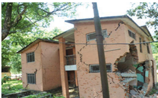
Ravaged Masonry Building
