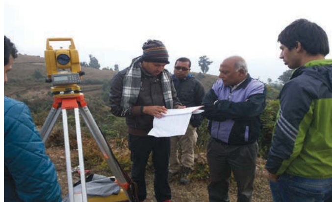
WAPCOS and NEA officials during Survey Mapping of Substations of Package 2 (Basantapur Substation)
