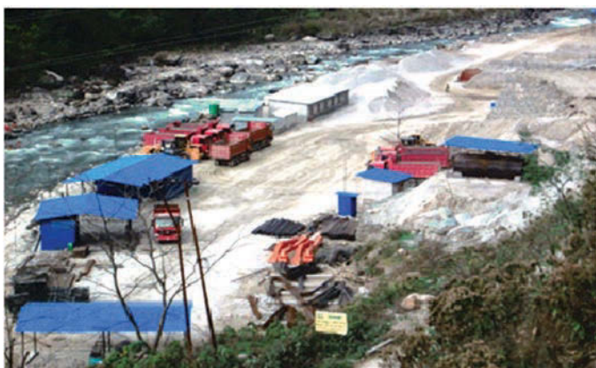
Aggregate Crushing Plant
