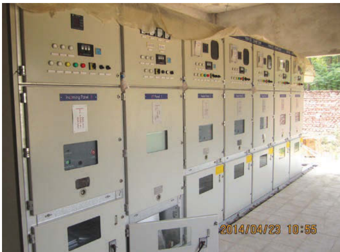
Latest 12 kV Indoor switchgears installed at different 33/11kV S/S
