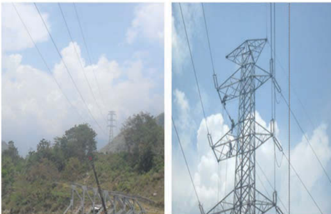
2nd circuit conductor stringing work under Middle Marsyangdi-Dumre-Lower Marsyangdi 132 KV Transmission line corridor
