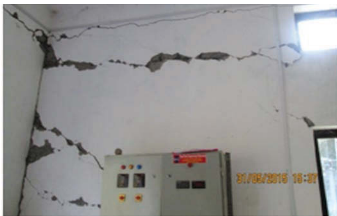
Damaged inside wall
