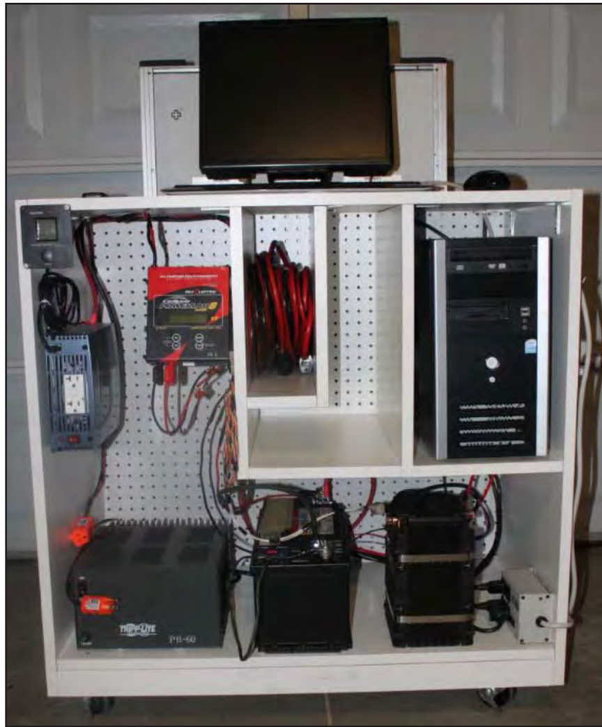
Figure 10. Mobile Energy Storage Unit, as Assembled
