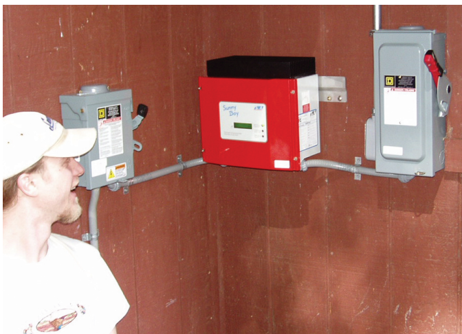
The inverter (red box) center is flanked by (gray) junction boxes each with a knife switch that can isolate power from the PV array and the main circuit panel. (Photo Credit: Marc Fontana)
