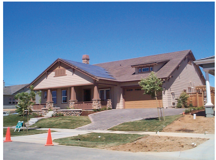
New single family housing projects like this in Livermore, California have upgrade options that include photovoltaic systems. This polycrystalline PV system is rated at 3.6 kW and is "grid connected". (Photo Credit: David Springer, Davis Energy Group).
