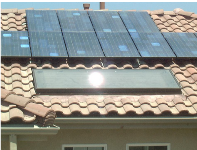
A solar water heating panel is installed below the PV array. (Photo Credit: Les Nelson, CAL SEIA)
