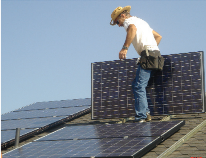
An installer adds a PV module into the array. (Photo Credit: Rodney Slaughter)
