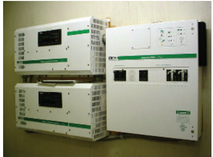
The inverters used in this system convert PV generated direct current to alternating current. (Photo Credit: Alan Wing)
