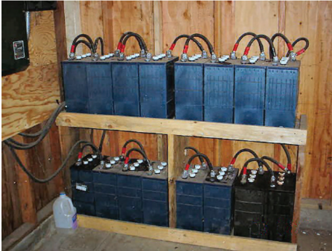
Batteries shown here in a well ventilated garage on wooden storage racks connected together in series and parallel. (Photo Credit: Alan Wing)
