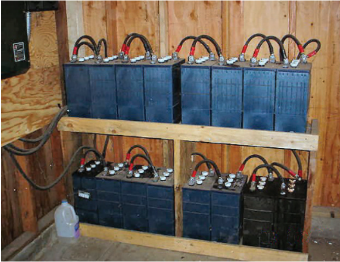
A bank of batteries similar to the one shown here would be used to back-up the PV system in off grid applications. (Photo Credit: Alan Wing)
