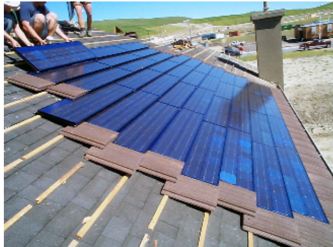
Centex Homes has built model homes in San Ramon, California. The homes were unveiled in the summer of 2004. The photograph shows PV tiles being installed on a tiled roof. (Photo Credit: Davis Energy)
