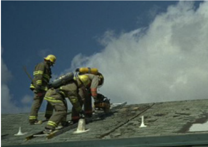
Roof vents pose a significant trip hazard to fire fighters conducting roof ventilation operations. (Photo Credit: Rodney Slaughter)
