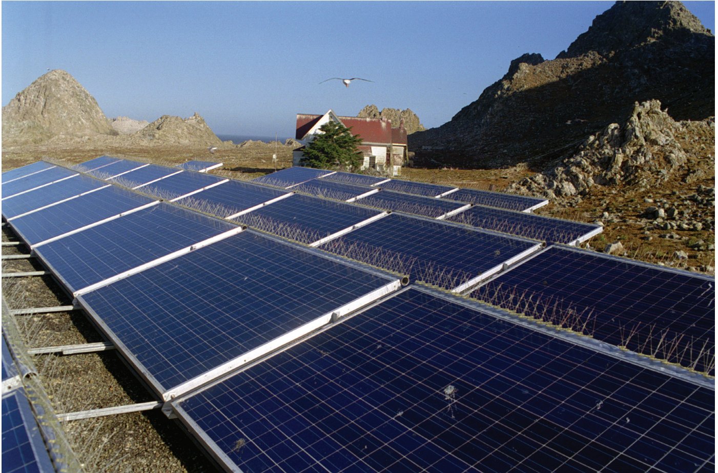
The US Fish and Wildlife Service needed a cleaner, quieter power source for this island 30 miles west of San Francisco. This reliable 9.1 kW photovoltaic system runs the facility that serves as a home for USFWS biologists who study the islands 6000 sea lions and thousands of birds. (Photo Credit: Farallon National Wildlife Refuge)
