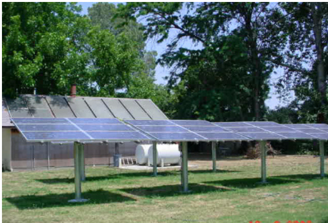
Fixed pole mounted PV system foreground with roof mounted PV modules and solar thermal modules on the roof in the background. (Photo Credit: Alan Wing)
