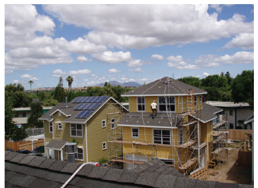
A multi-family housing development in Livermore, California is outfitted with photovoltaic modules. (Photo Credit: Marc Fontana).
