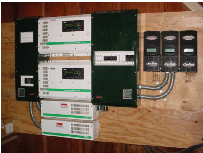
The controller monitors the electricity entering and exiting the back-up battery system. (Photo Credit Alan Wing)
