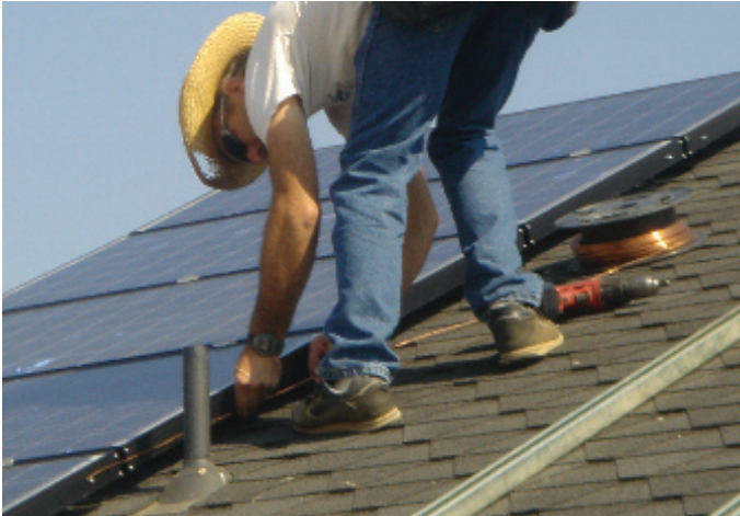
Installer is connecting a ground wire to each module in the PV array. (Photo Credit: Rodney Slaughter)
