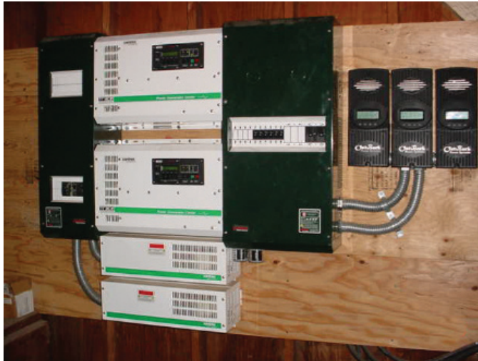
The battery controller shown here was used in an off-grid PV system. (Photo Credit: Alan Wing)
