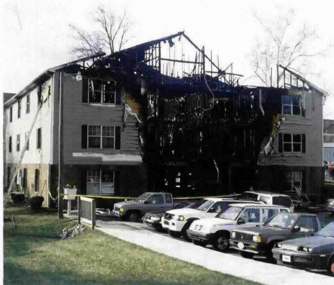
Four people died in this apartment fire in North Carolina. The cause was arson.
