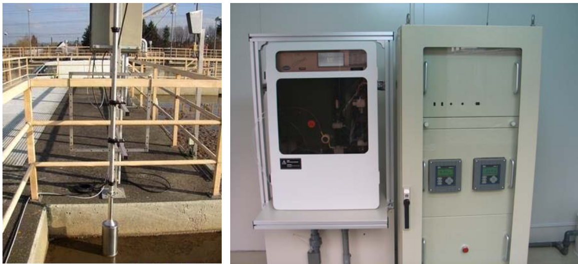
Figure 2-4: Online Monitoring Facilities in Wastewater Treatment Plant
