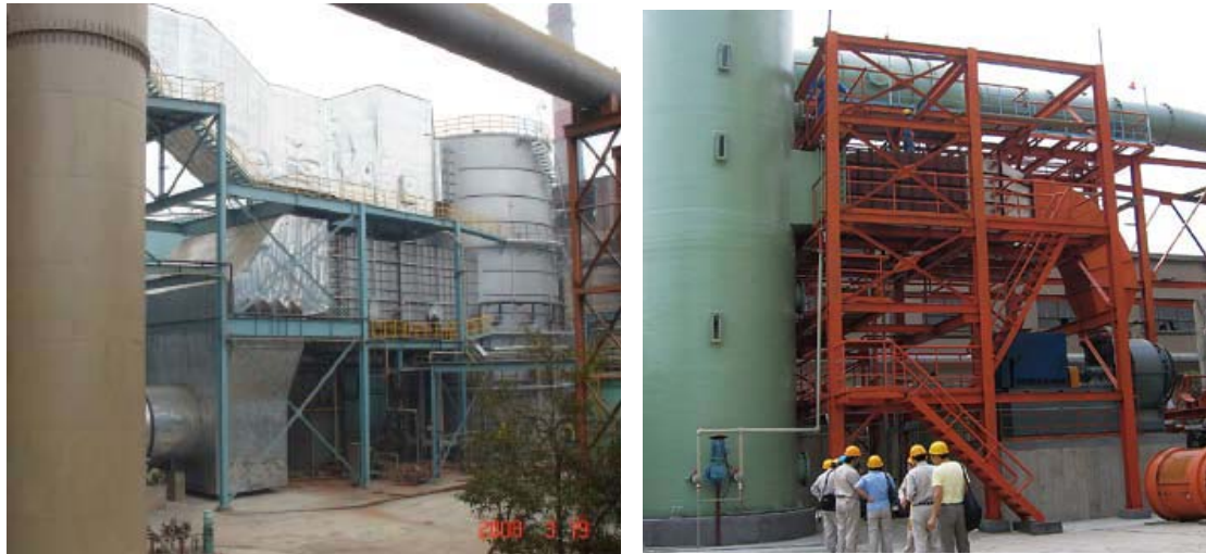
Figure 2-16: Desulphurization Facilities in Baosteel Power Plant
