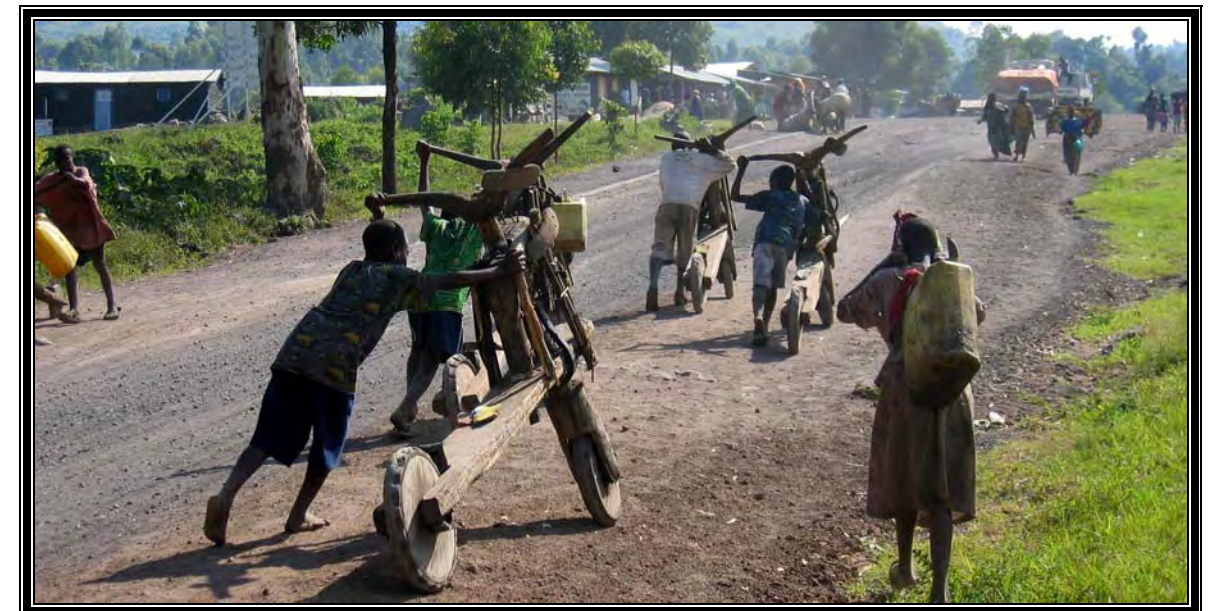
A section of the Goma-Rumangabo asphalt road was damaged by the 2002 volcano lava flow
