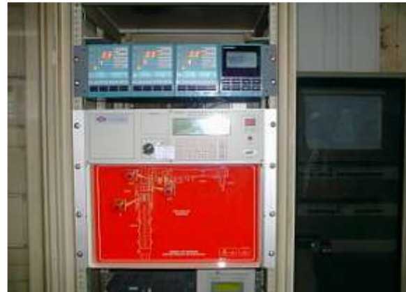
Remote display in Control room
