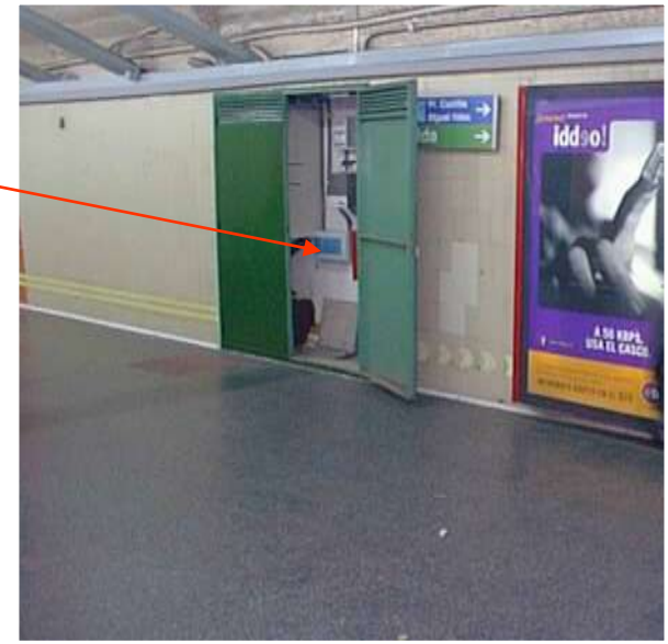
ASD inside Electrical cabinet
