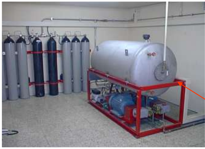
Every station is equipped with one high-pressure water mist cylinder room
